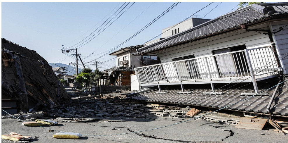
Figure 2: Buildings damage on sloping ground due to earthquake
