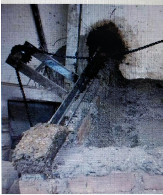
Fig. 3.6 Pulley inclined at 45° with vertical and girder fixed on the top of the wall of pit {DTU thesis}[4]
