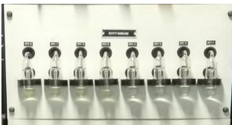
Figure 2.13 Safety bubbler showing no bubbles
