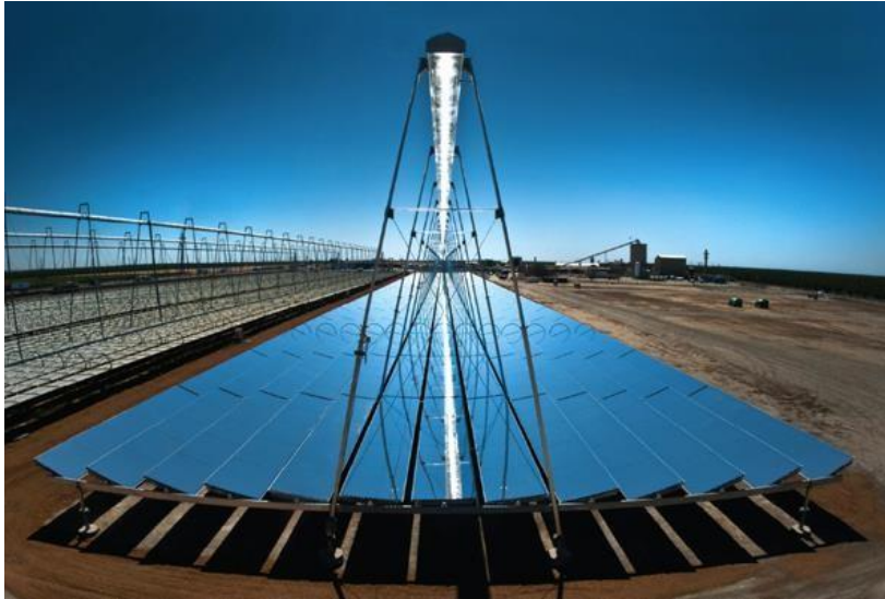
Figure 8: Kimberlina linear Fresnel power plant (California) [8]
