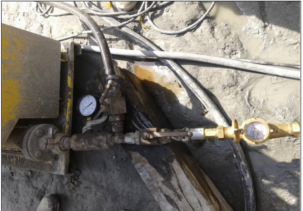
Fig 3.23 Pressure Gauge and Water Flow Meter
