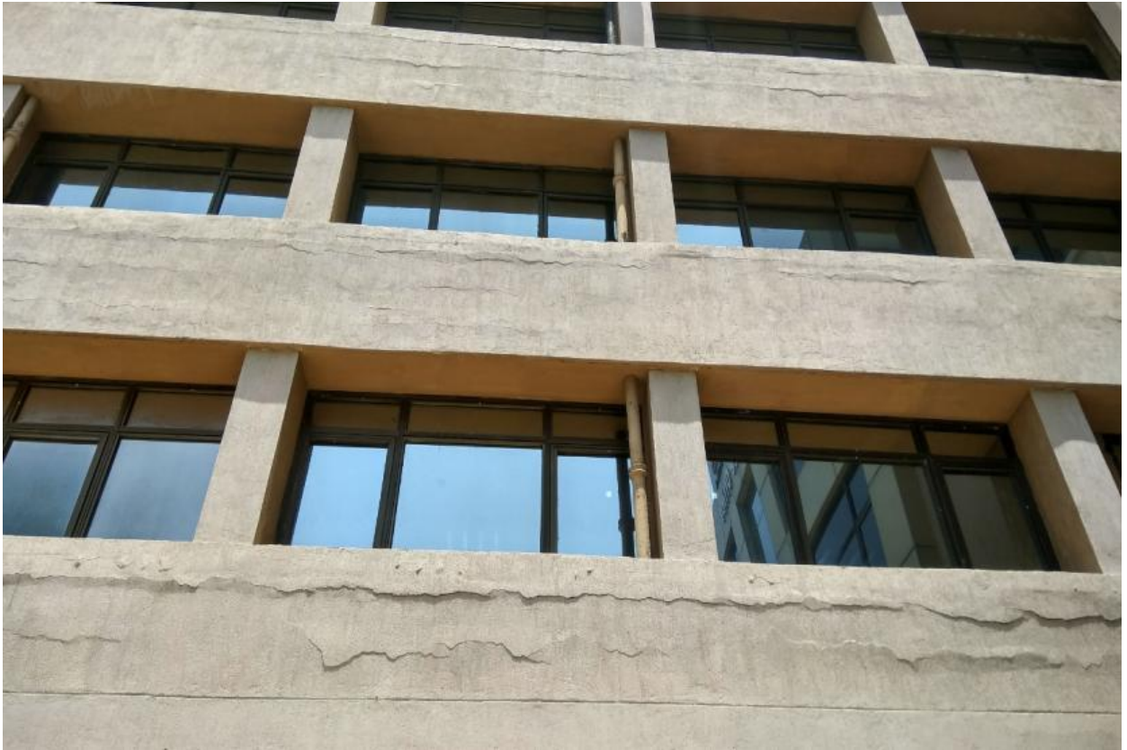
Fig. 8(d):- Showing Cracks in plaster and probably in beam
