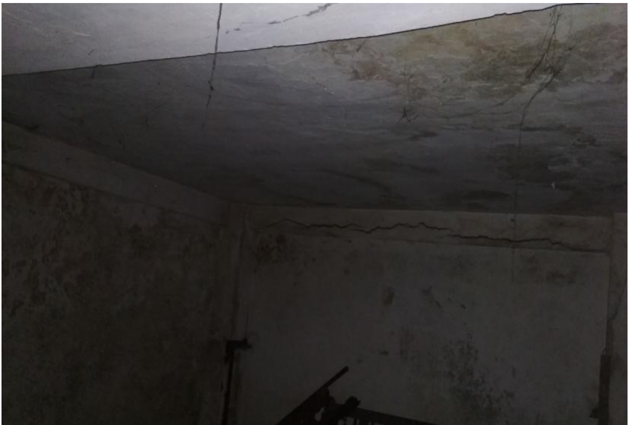
This Portion requires re-construction can't be repaired
