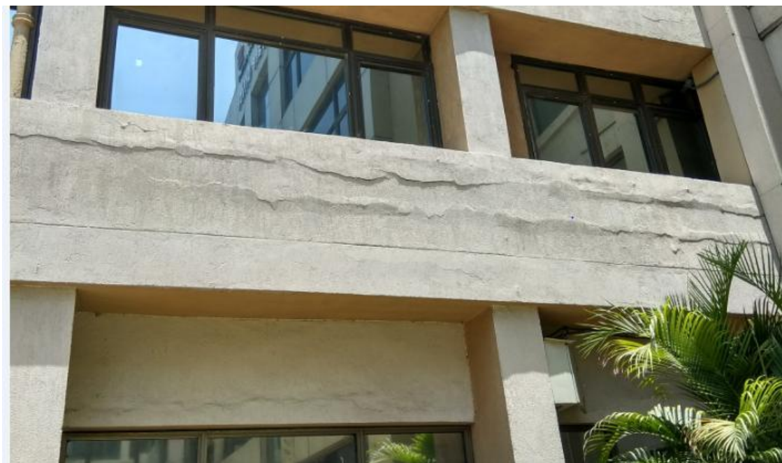
Fig. 8(b) Showing Cracks in plaster with some swelling
