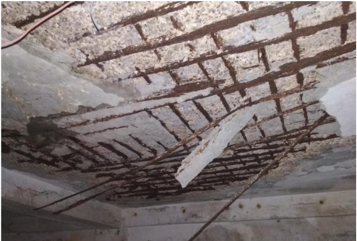
This Portion requires re-construction can't be repaired
