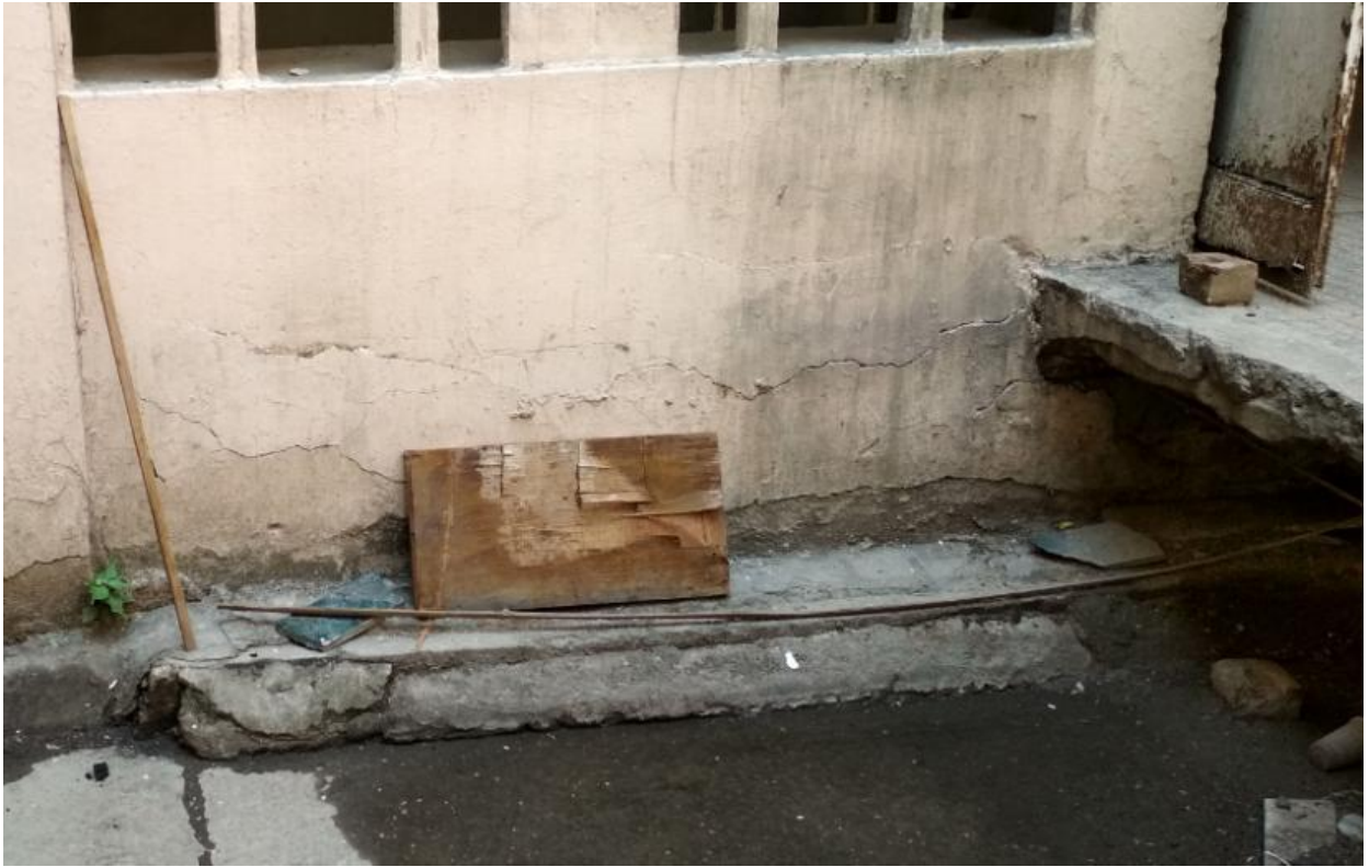
This Portion requires re-construction can't be repaired
