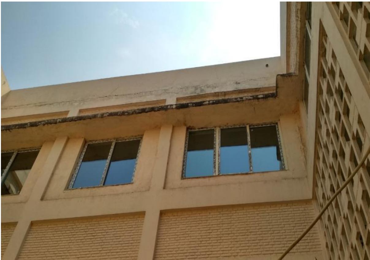
This Portion requires re-construction can't be repaired
