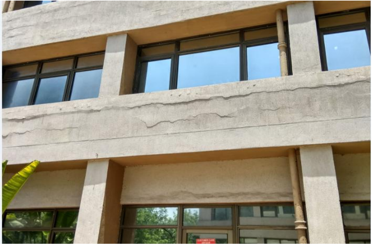
Fig.8(c):- Showing Cracks in plaster and probably in beam
