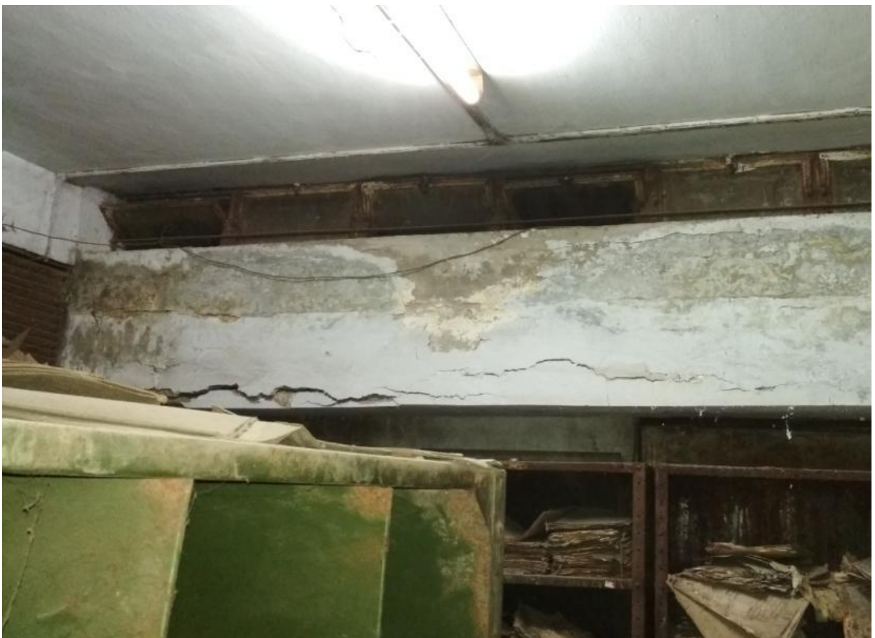
This Portion requires re-construction can't be repaired
