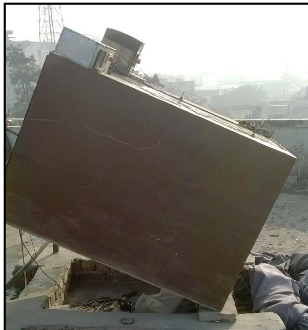
Fig. 3.14 Roof top installed collector
