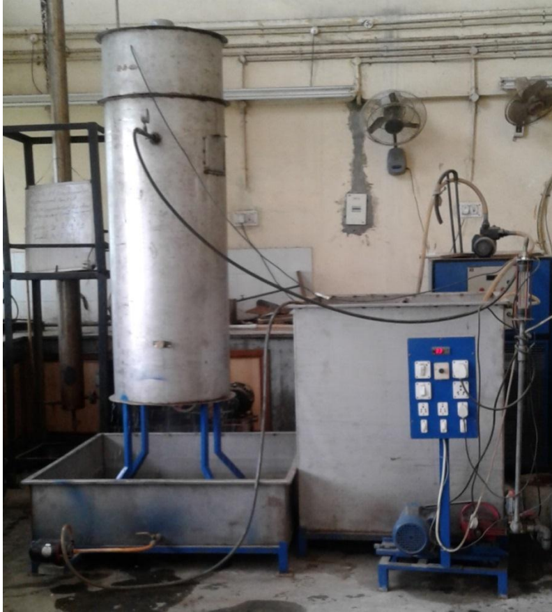
Figure 3.3 Actual shower cooling tower
