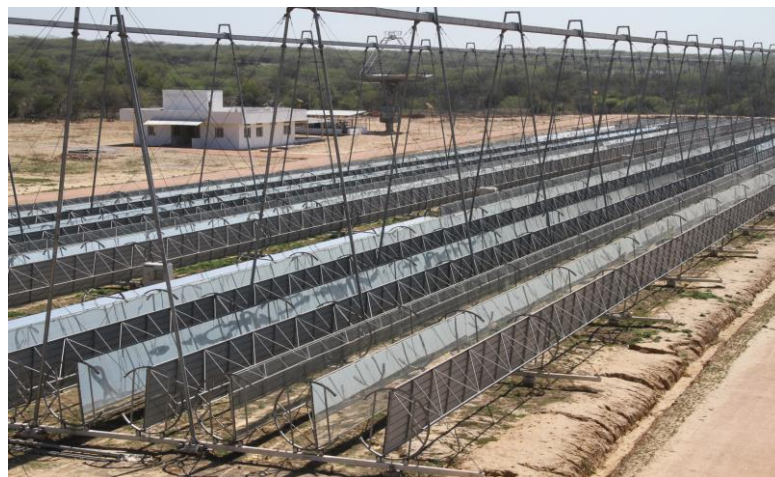
Figure 2.3 A typical linear fresnel reflector installed at NISE
