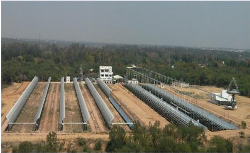
Figure 2.2 1 MW solar thermal power plant installed at NISE
