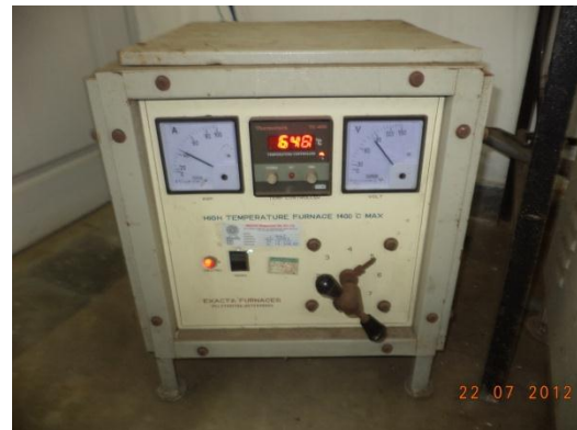
Furnace Voltage Stabilizer
