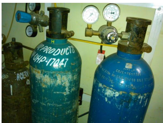
Acetylene and Oxygen gas Cylinders
