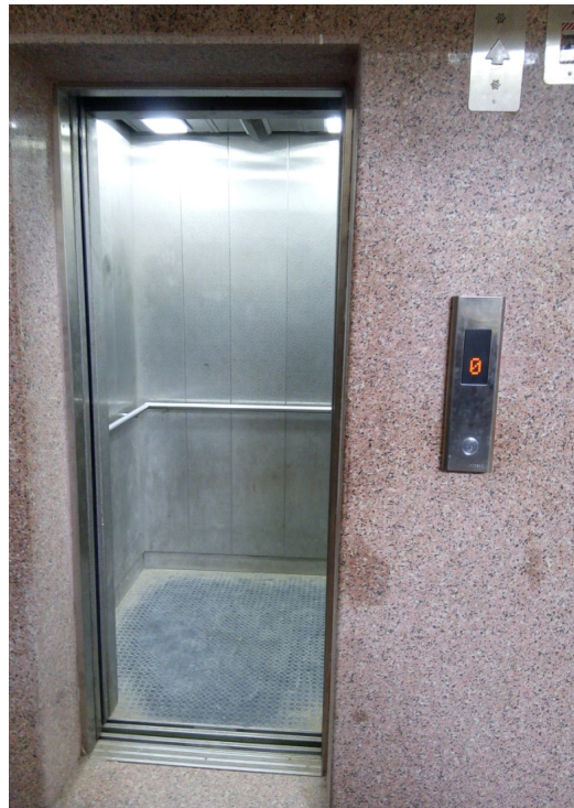
Figure 3.53 Lift provided in Electronics and Communication Engineering Department
