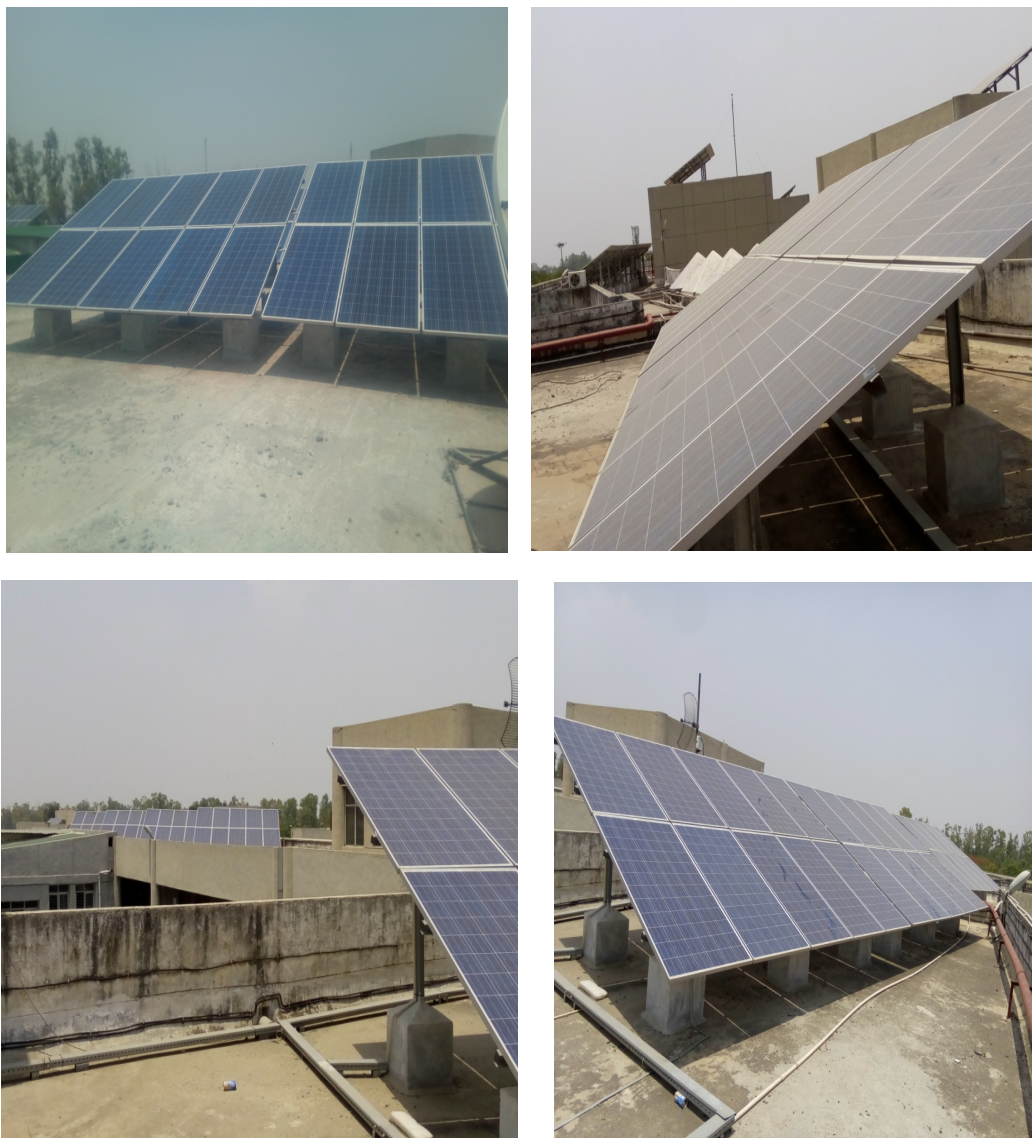
Figure 3.22 Solar Panels Installed in various Engineering Departments of DTU.
