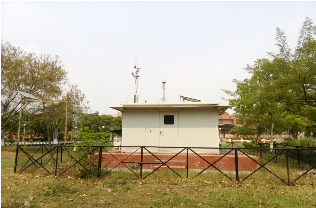
Figure 3.35 Ambient air quality monitoring station at DTU installed by CPCB, Delhi
