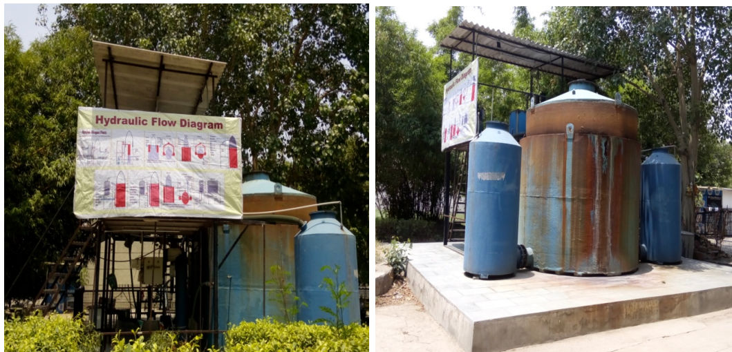
Figure 3.48 Rocket Biogas Plant to treat organic wastes generated in the DTU into biogas.
