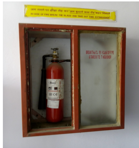
Figure 3.31 Fire extinguisher used in Electrical Engineering Department
