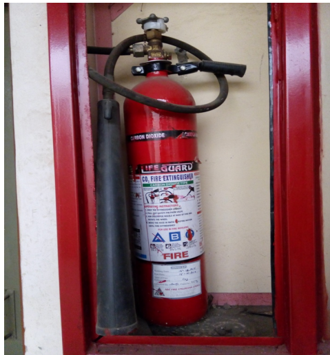
Figure 3.30 Fire extinguisher used in Computer science and I.T Engineering Department
