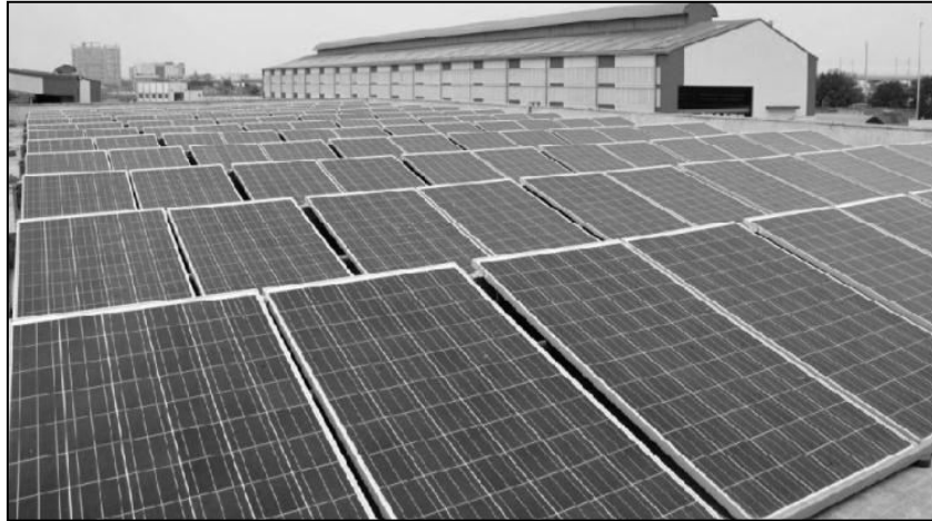
Fig. 3.3 500kW P solar photovoltaic plant at Dwarka
