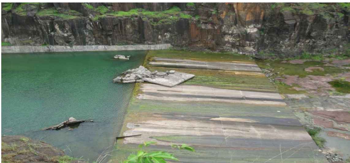
Fig. 2.2 View of dislodged RCC panels in Bhama Askhed dam EDA
