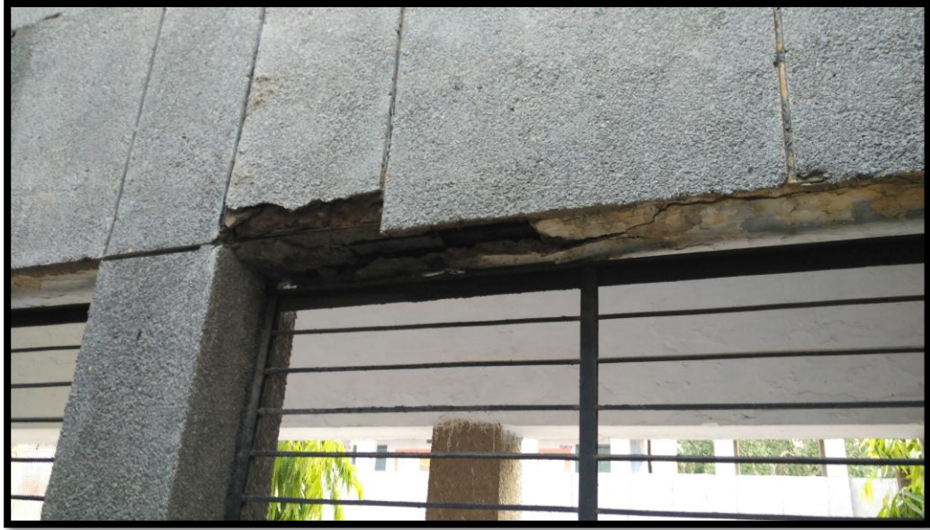
Picture 7: Spalling of concrete in the beam
