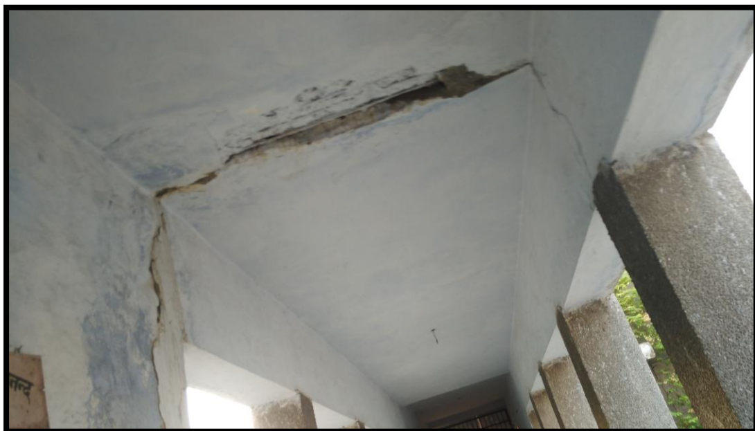
Picture 8: structural Crack in the corridor at 1 st floor
