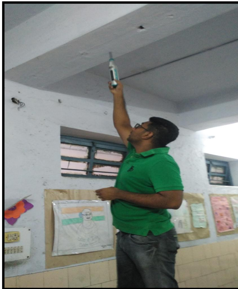
Picture 16: RH Reading of beam in block D
