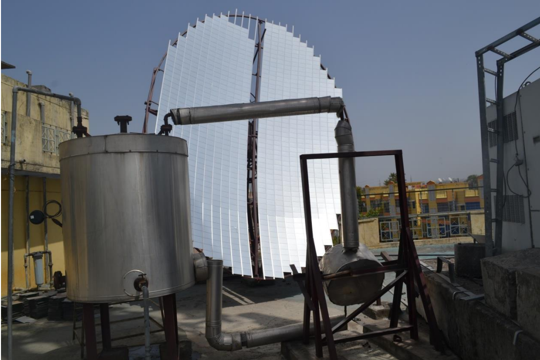
Fig.4.7: Feed water storage tank with separate Scheffler Dish for pre heating water
