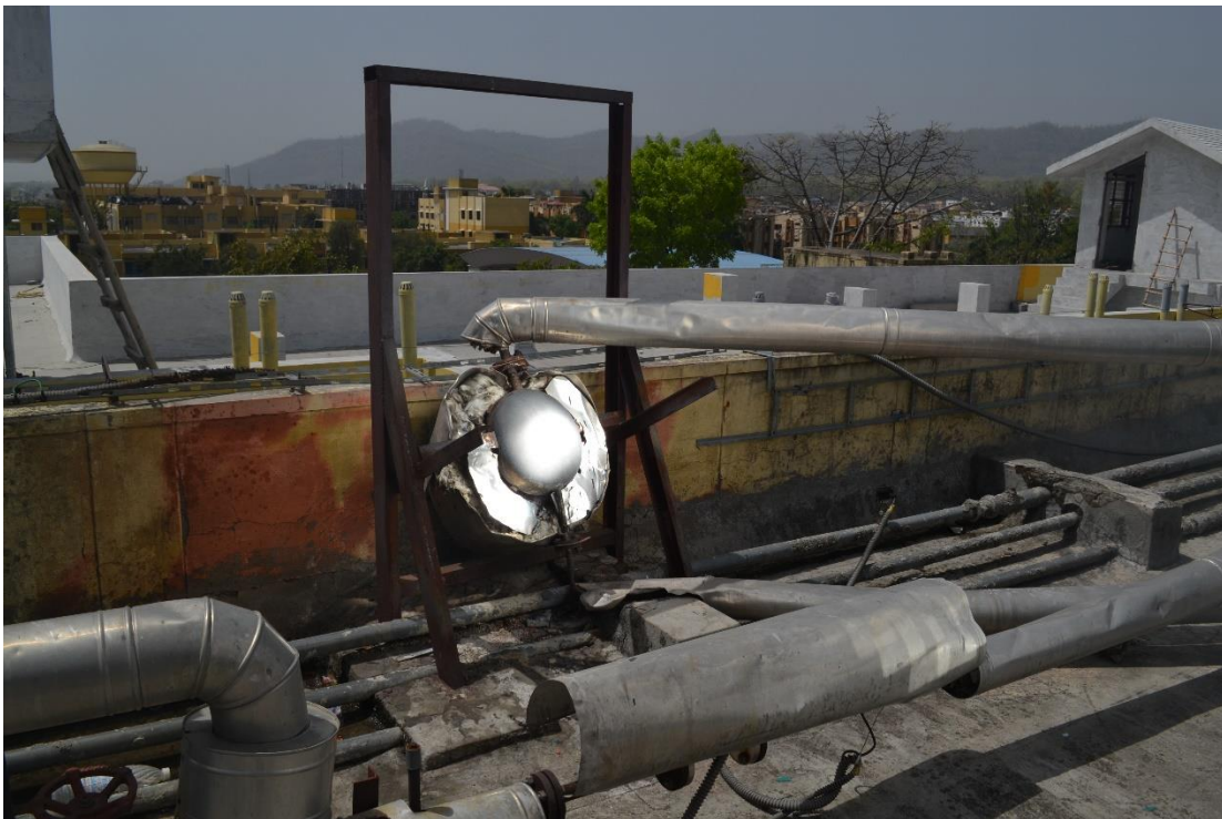
Fig.4.8: Receiver with supporting structure and inlet and outlet pipes
