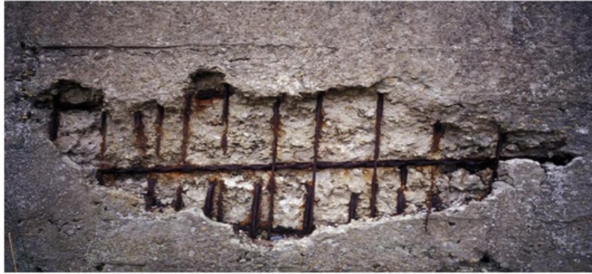
Figure 4: Spalling of concrete slab due to corrosion [1]
