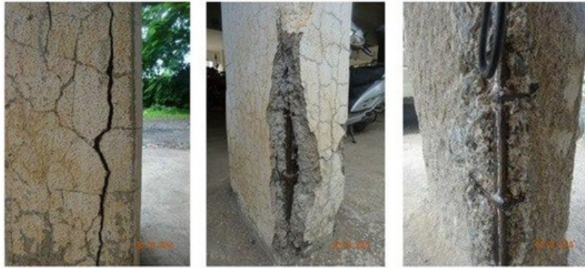
Figure 5: Cracks formed in RCC Column, Rebar gets exposed [2]
