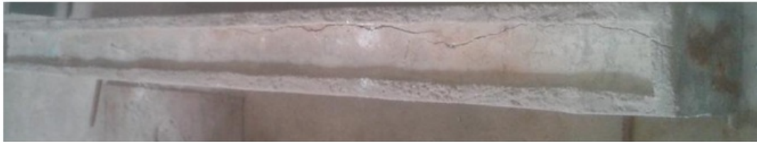
Figure 9: - Cracks on beam due to corrosion of steel
