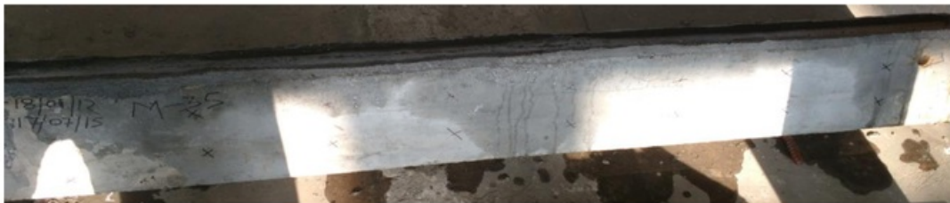
Figure 17: - Condition of beam after curing for 28 days
