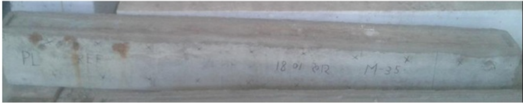
Figure 8: - Beam member before repairing
