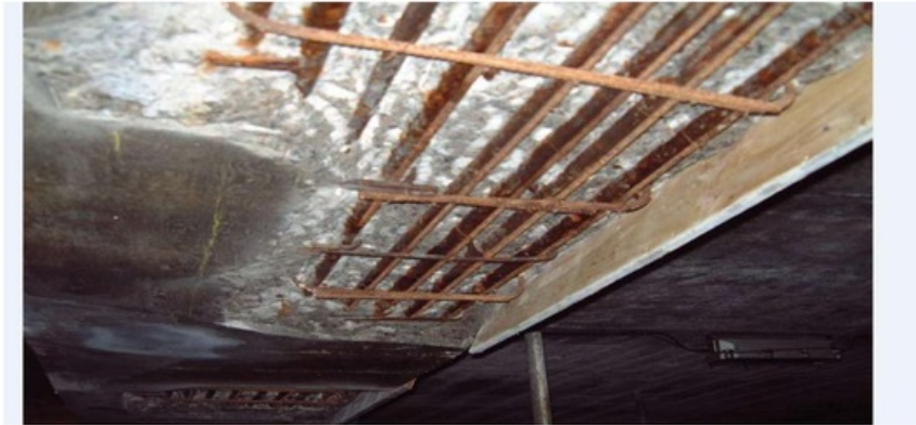
Figure 6: Corrosion of rebar in bridge beam [3]
