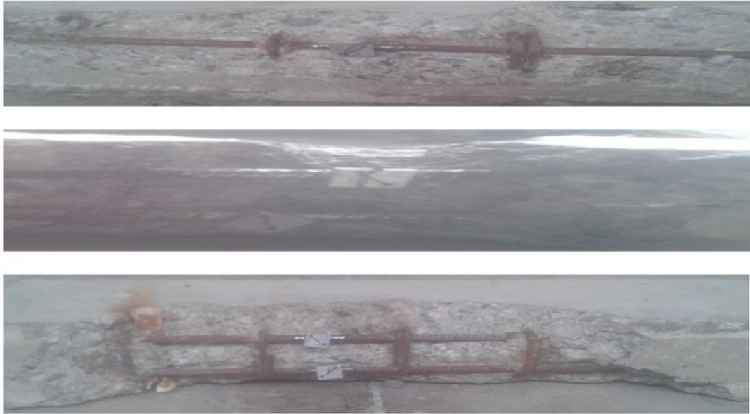
Figure 13: - Attaching Zinc Blocks to the rebars in patch work of Beam member
