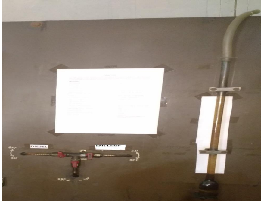
Plate.3.9: Fuel measurement system
