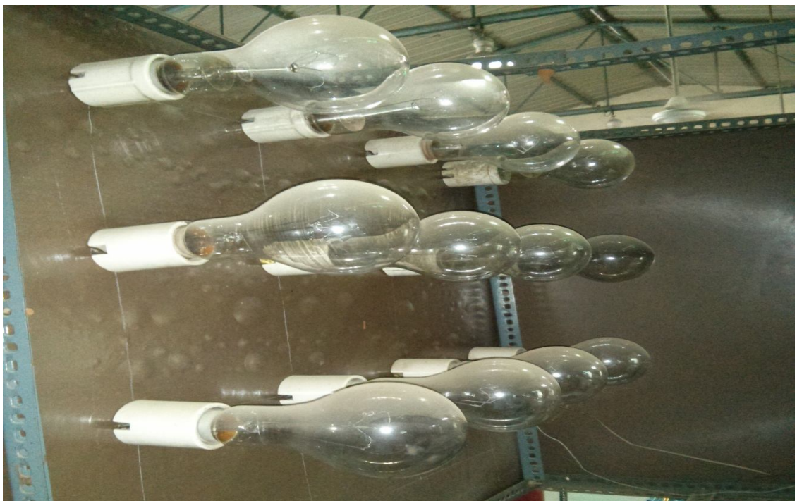
Plate 21 Load Bank for the Experimental Setup
