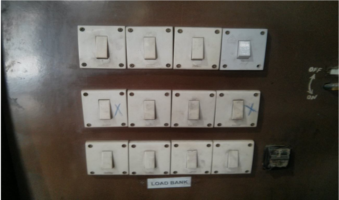
Plate 22 Load Bank Switches mounted on the front of control panel
