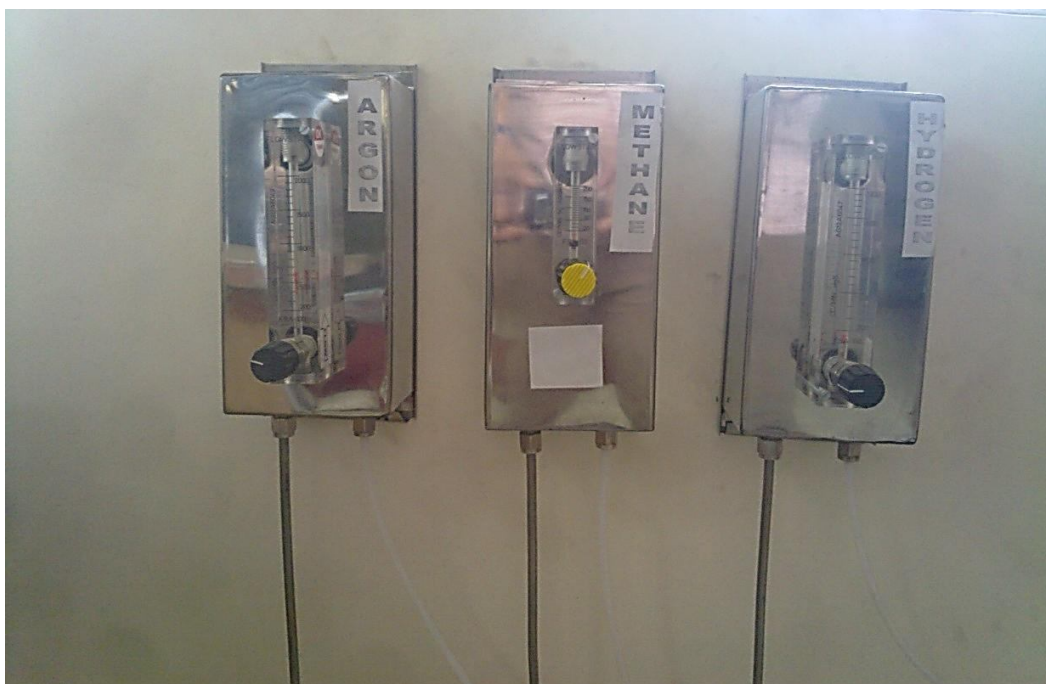
Plate 4 Gas Cylinder Controllers
