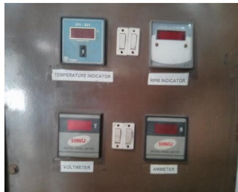
Plate 18 Control panel meters
