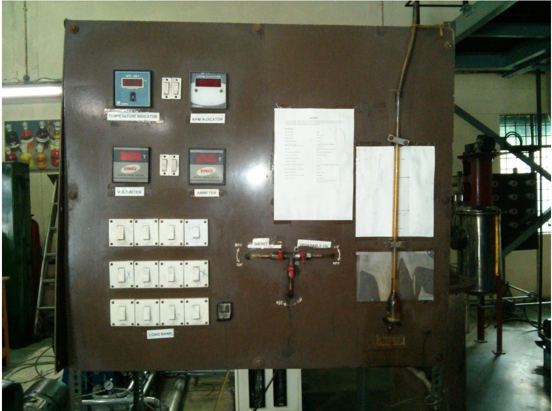
Plate 20 Control panel for the experimental setup
