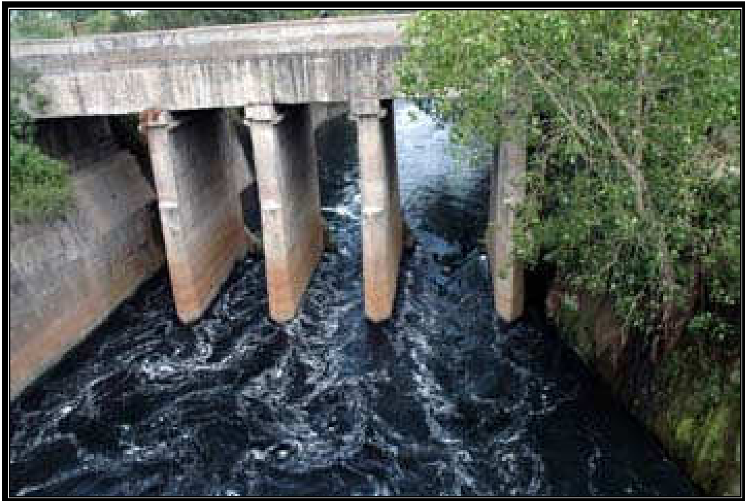
FIGURE 5.2: Najafgarh drain Swirl under a bridge on the way to River Yamuna
