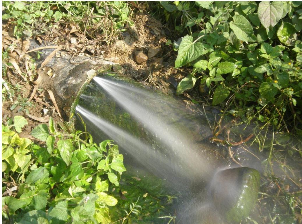
Fig 4.13: Photograph showing leakage of Ductile Iron pipe from the joint.
