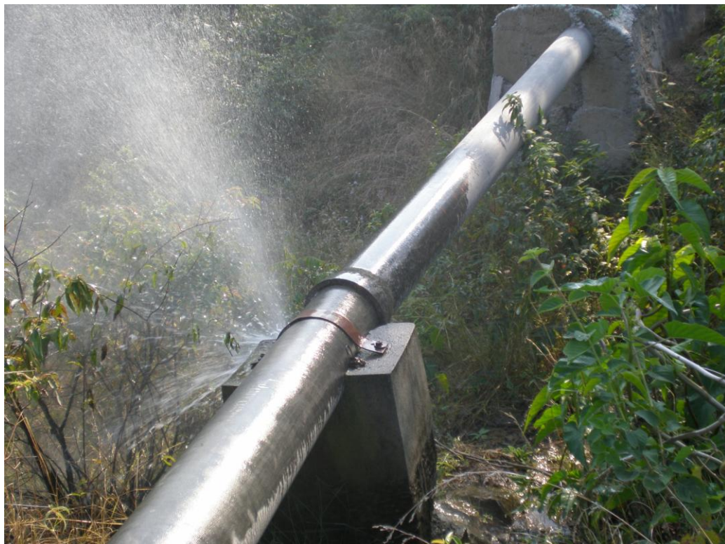
Fig 4.12 Photograph showing leakage of Ductile Iron pipe at the joint.
