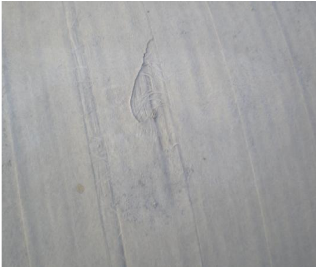
Fig 4.11: Photograph showing disintegration of GRP fibres.
