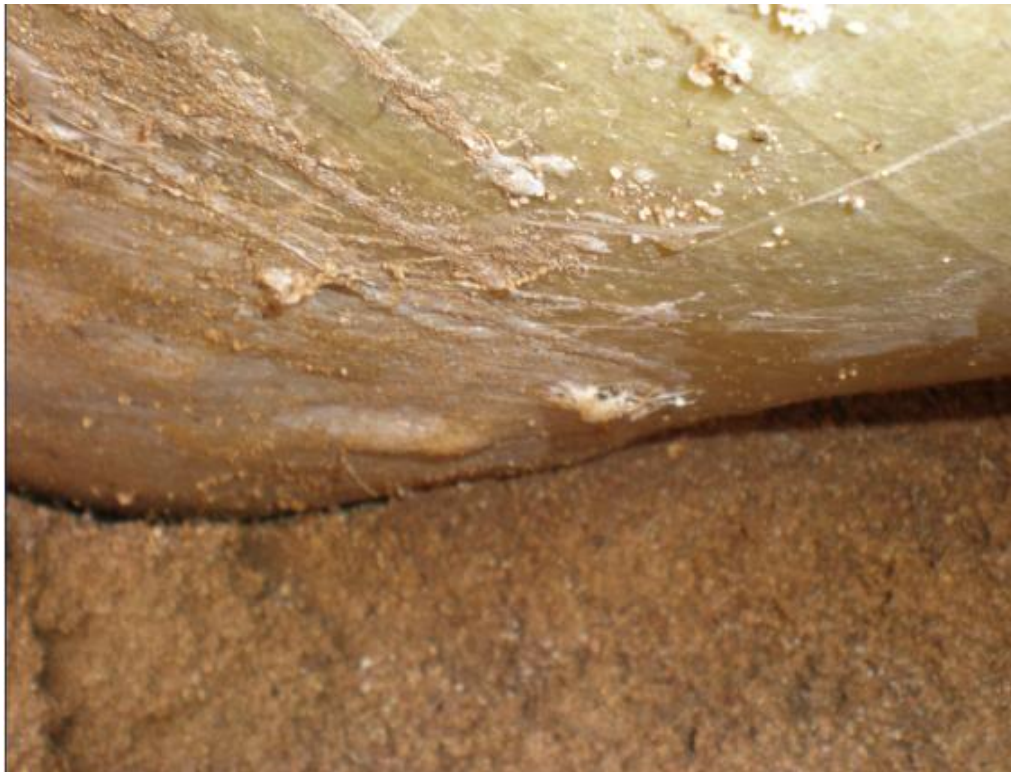
Fig 4.8: Photograph showing disintegration of GRP fibers subjected to high internal pressure.
