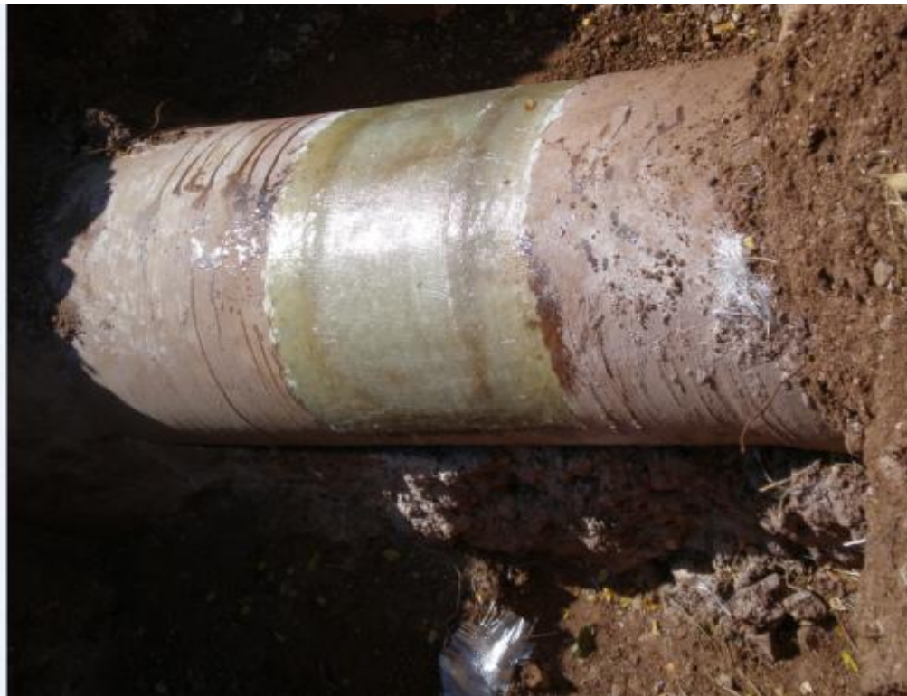
Fig 4.6: Photograph showing leakage in repaired GRP pipeline.
