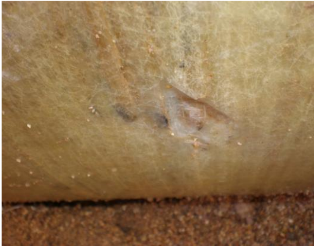
Fig 4.7: Photograph showing cracks in pipe wall due to presence of sharp object in the surrounding.
