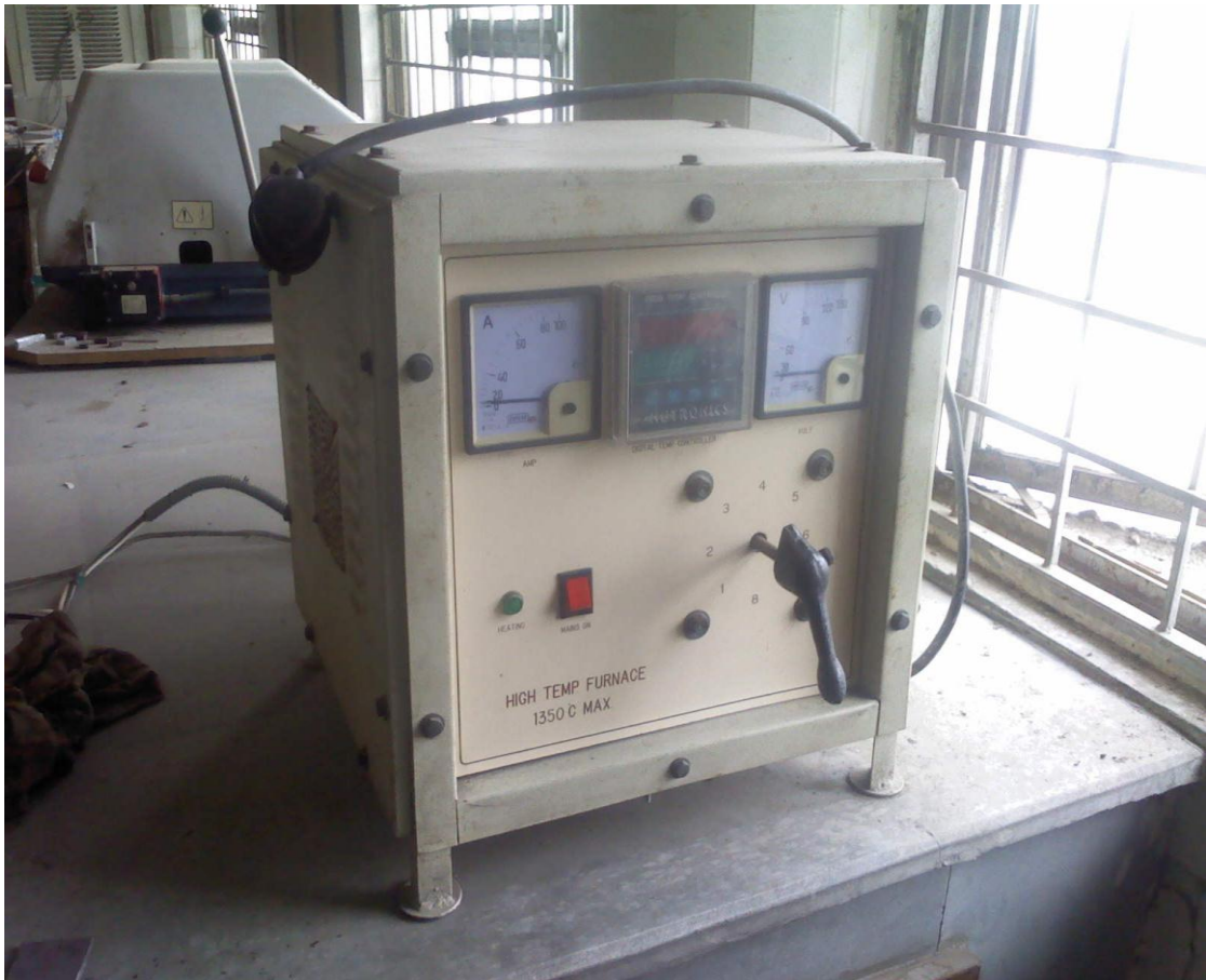
Fig. 3.3 Temperature control unit of furnace
