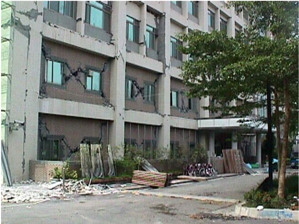
Figure – 1: Effect of earthquake in brick infill
