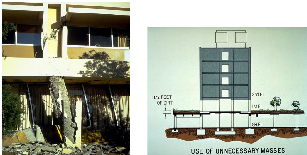
Figure1: Olive View Hospital, San Fernando, California partial View of the 5-story Medical Treatment and Care Unit [2]
