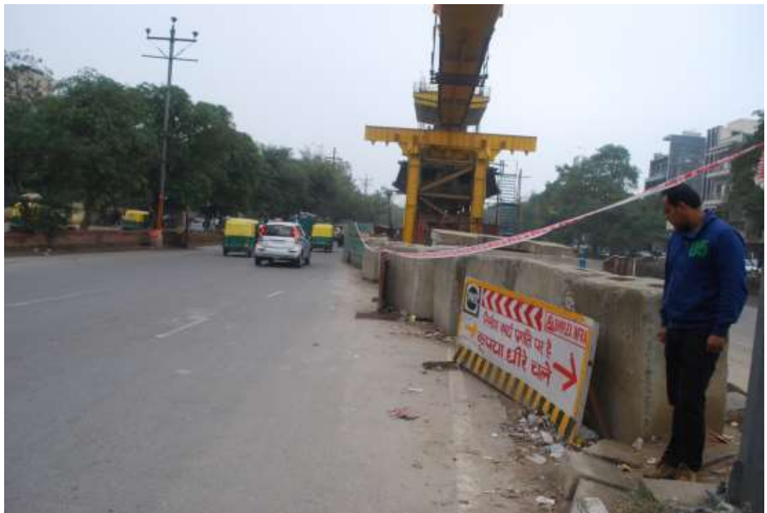
Figure 5: Misleading signboard, No informatory or Warning signboards
