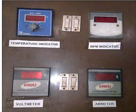
Plate 3.12 Control Panel (Indicator & Meter)
