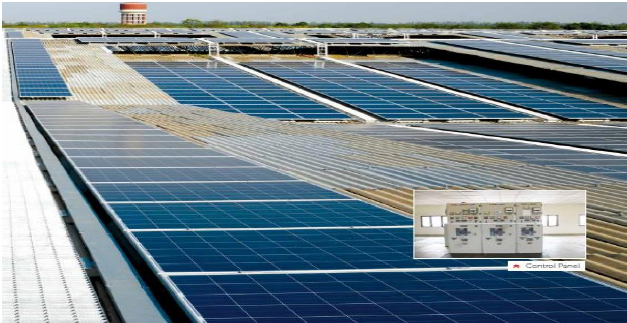
Fig 2.1: Rooftop installation of solar rooftop PV project of 7.524 MWp capacity at RSSB [31].
