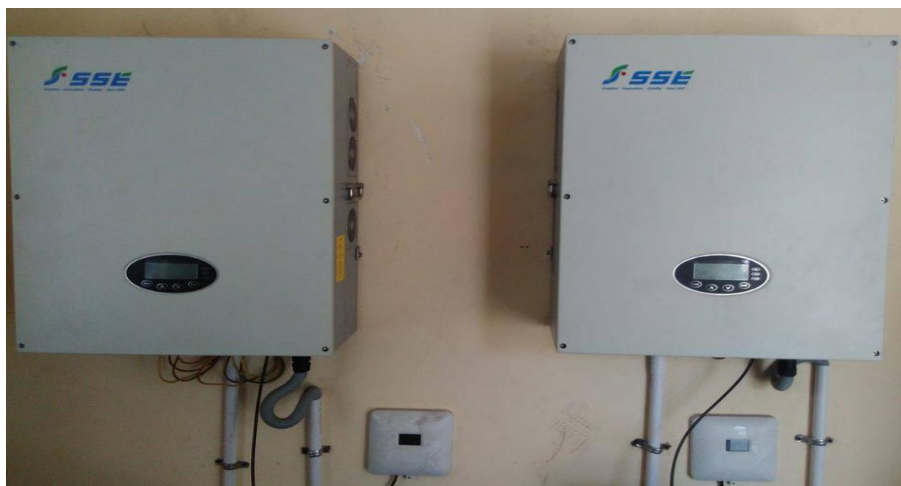
Fig5.5: Actual picture of installed two 20 kW SSE inverters at 40 kW SPV system at DTU [30].
