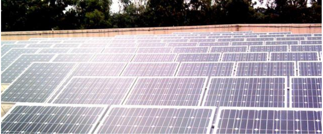
Fig 7.2: Actual installed photograph of 25 kW SPV system at Sewa Bhawan, New Delhi.
