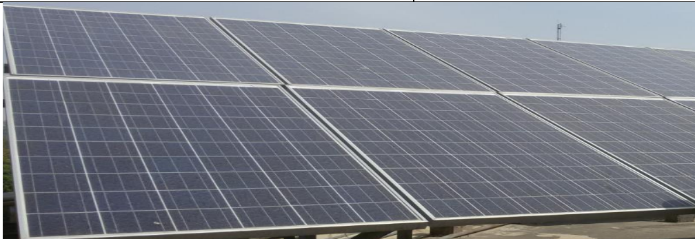
Fig 5.4: Actual picture of installed PM250 photon energy modules at 40 kW SPV system at DTU.
