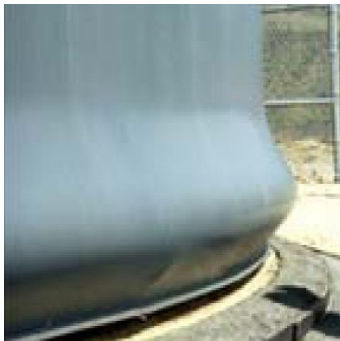
Figure 2.2: Elephant foot buckling of broad tank[22]
