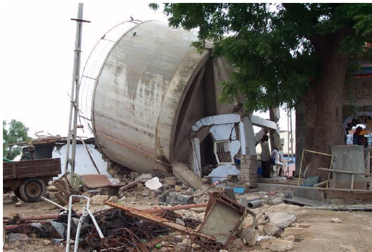
Figure 2.1: Collapsed elevated tank in Bhuj(India)[22]
