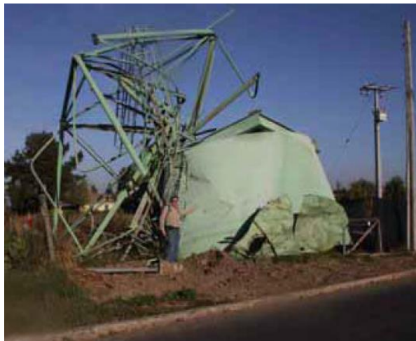
Figure 2.6: Typical collapsed small steel water tank[22]
