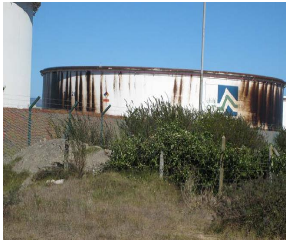
Figure 2.5: Oil tank sloshing spill over the tank[22]
