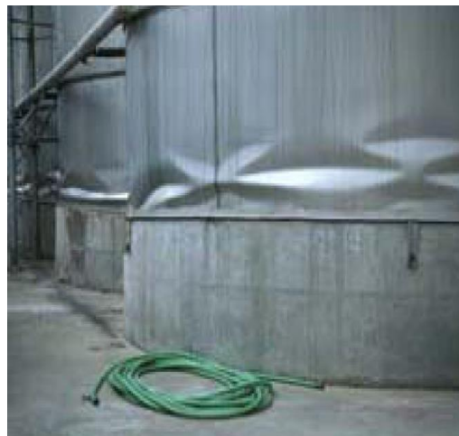
Figure 2.3: Diamond buckling in slender tank[17]
