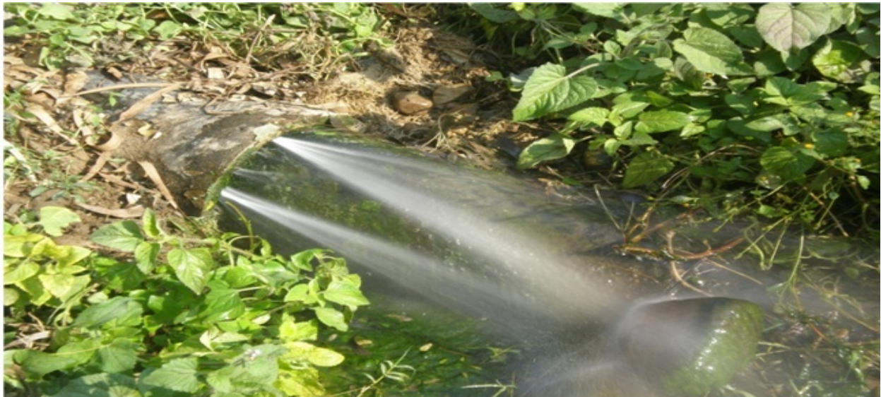
Fig 4.8 Photograph showing leakage of Ductile Iron pipe at the joint
