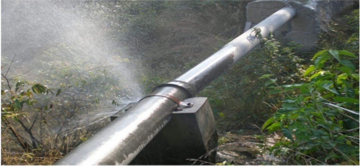
Fig 4.9: Photograph showing leakage of Ductile Iron pipe from the joint.
