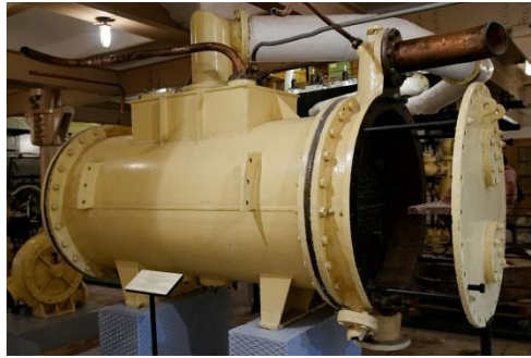
Fig. (7). Surface Condenser
