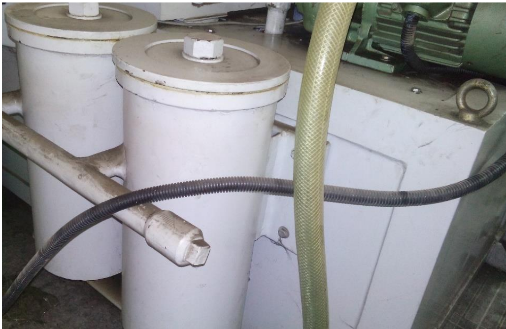
Figure 16 - Dielectric reservoirs and pump
