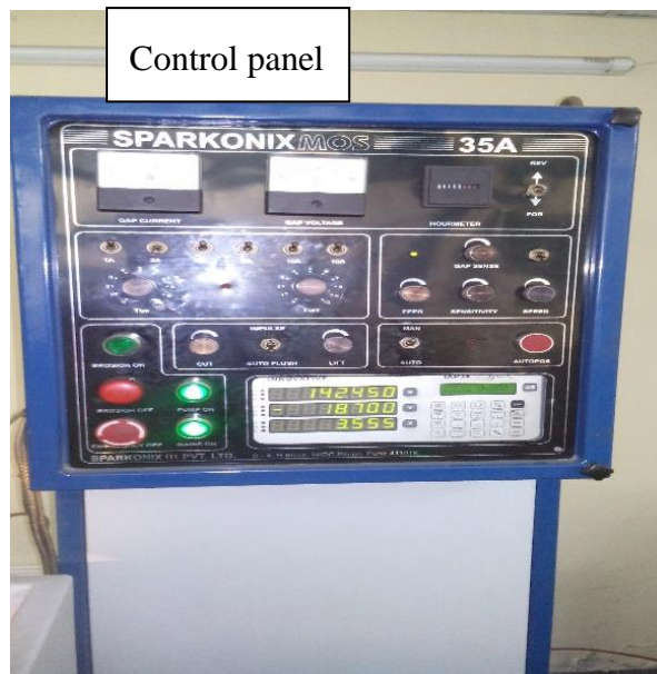
Figure 17 - Control panel and display unit
