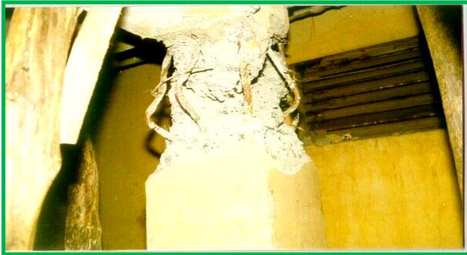
Figure 9*[1]: Damage to columns in the soft storey of a framed building during earthquake
