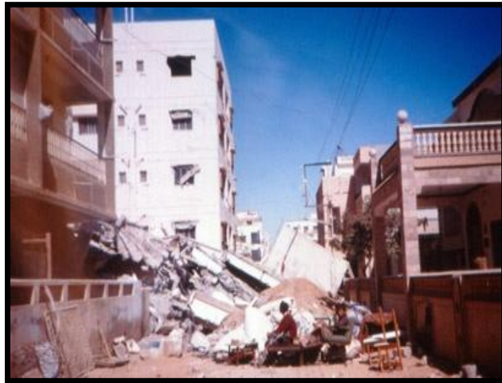
Figure * 4[2]: Collapse of a framed building due to failure of ground floor columns in Bhuj, 2001
