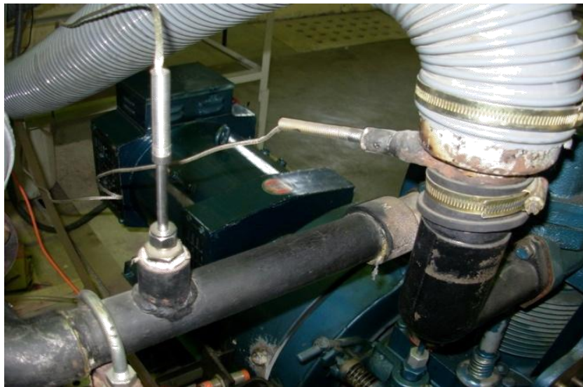
Plate 3.16: Temperature Measurement Arrangement
