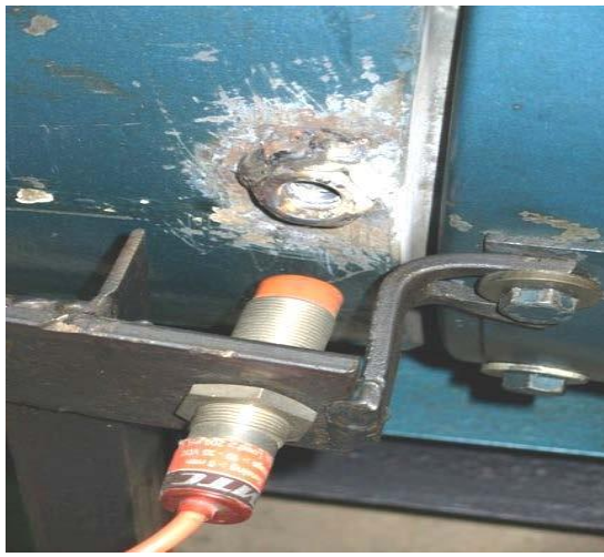
Plate 3.15: Engine Speed Measurement
