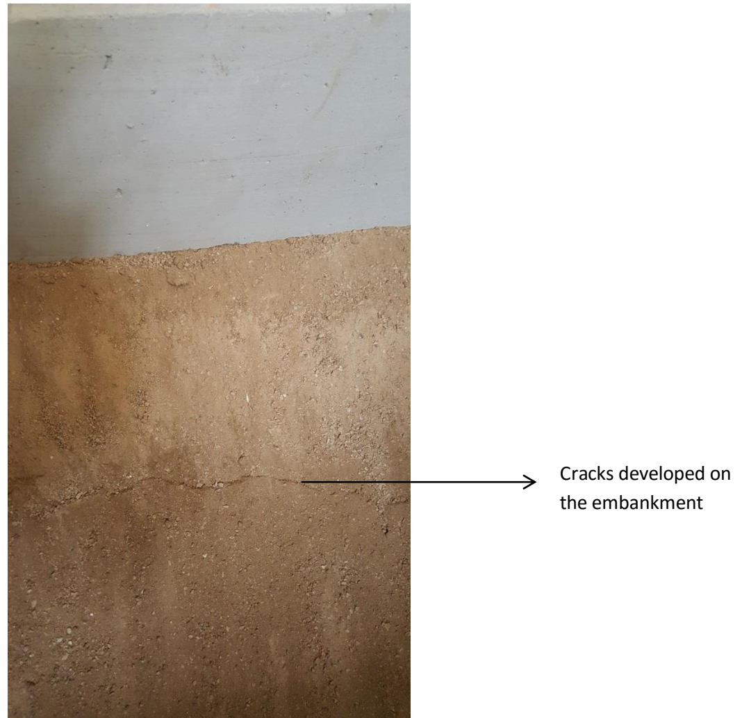
Figure 4.7a. Cracks Developed due to Loading on Embankment Without Micropiles
