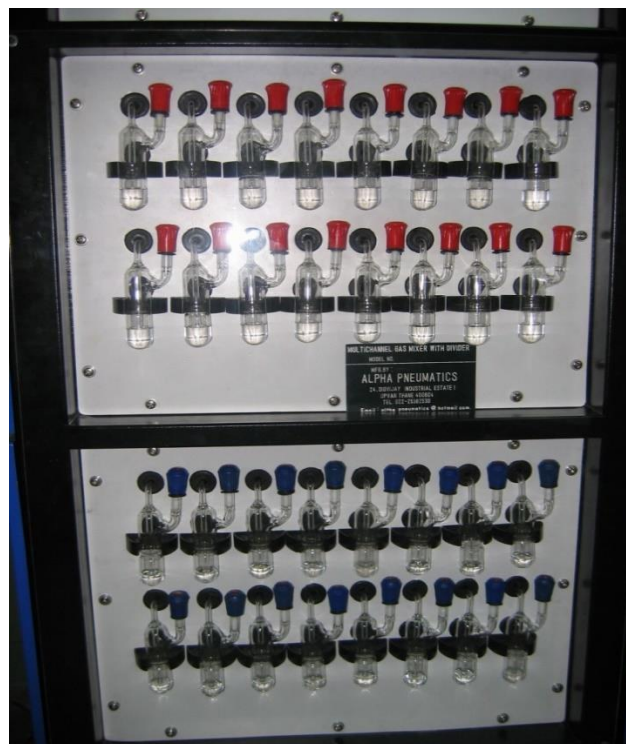
Fig 2.13 Safety and Isolation Bubbler unit
