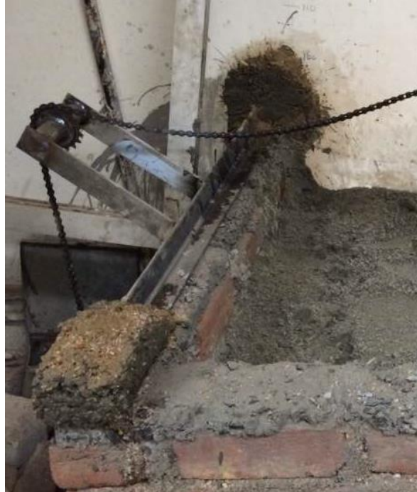
Fig3.4: girder fixed on top of brick wall and pulley inclined at 45° with vertical
