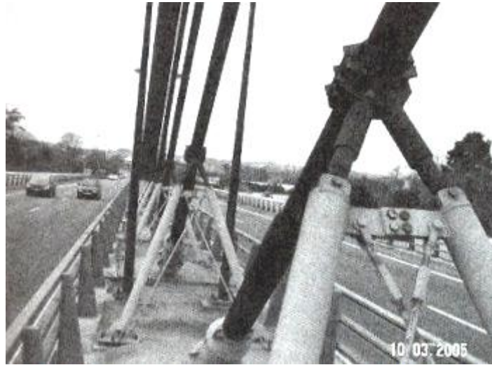
Figure.5.5. (a)– Hydraulic damper at Iroise.
