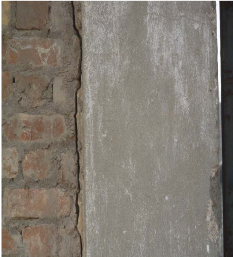
Fig. – 4.10 Original construction defects
