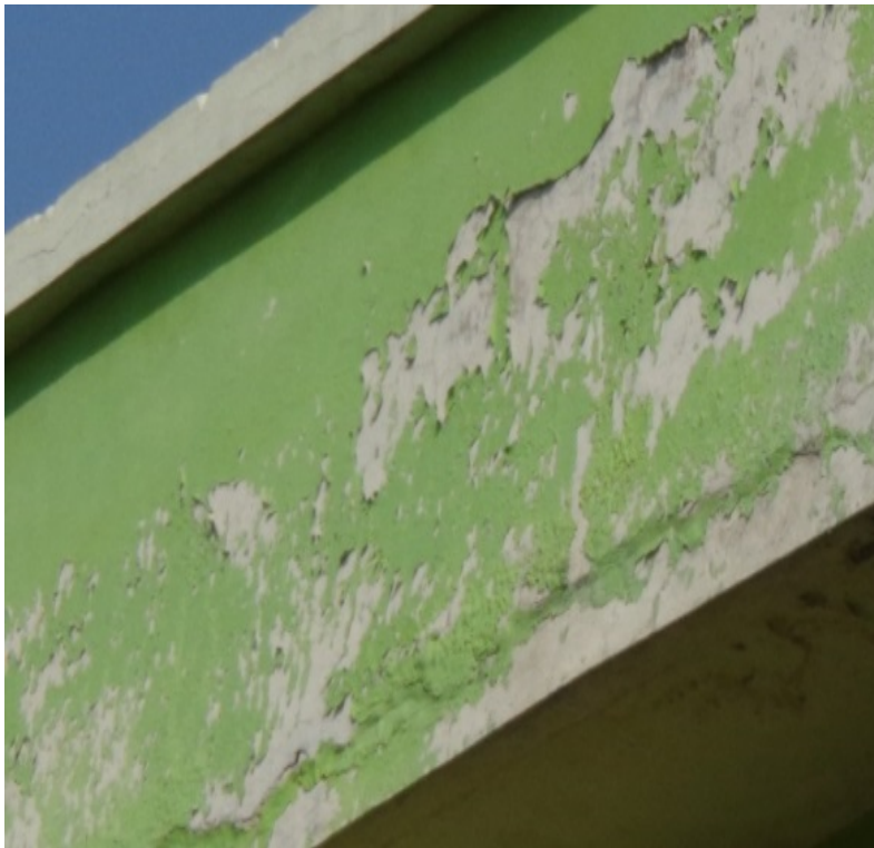
Fig.-4.15 Peeling of paint.
