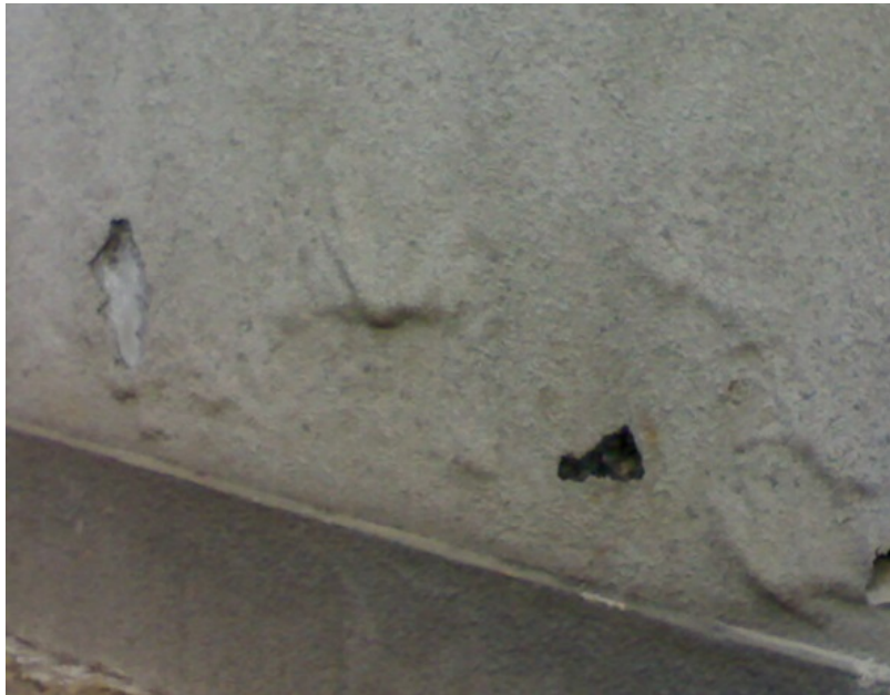
Fig.-4.14 Blistering of paint
