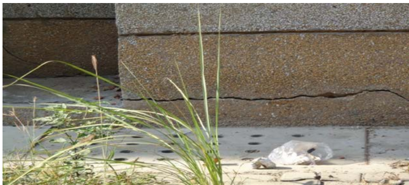
Fig. - 4.3 Horizontal crack at plinth level
