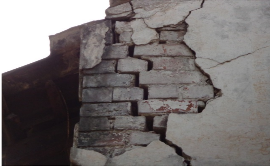
Fig. - 4.4 Major vertical crack in brick wall
