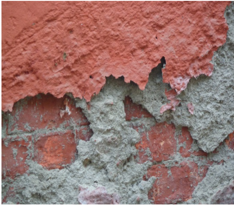
Fig.4-13 Plastering deterioration due to salt effect
