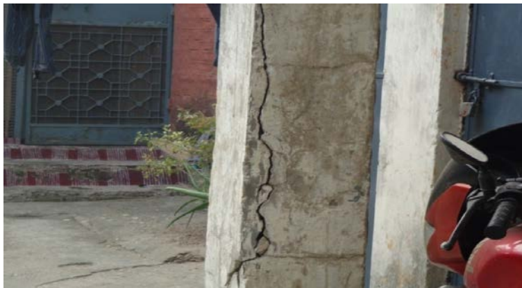
MEDIUM DETERIORATION OF RCC COLUMN
