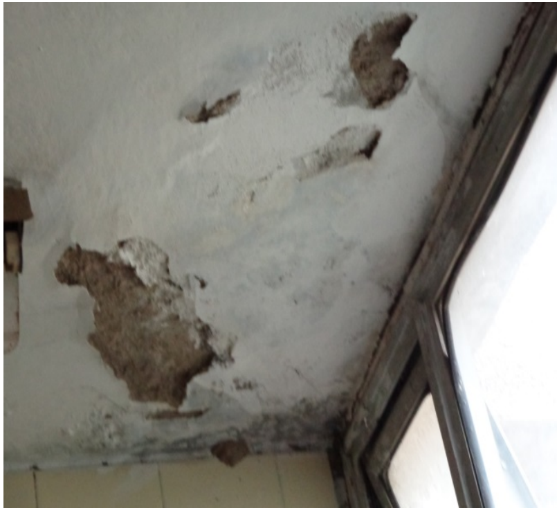
Fig.-4.11 Plastering deterioration due to dampness under slab
