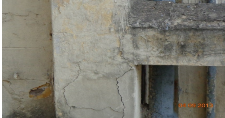
MINOR DETERIORATION OF RCC COLUMN
