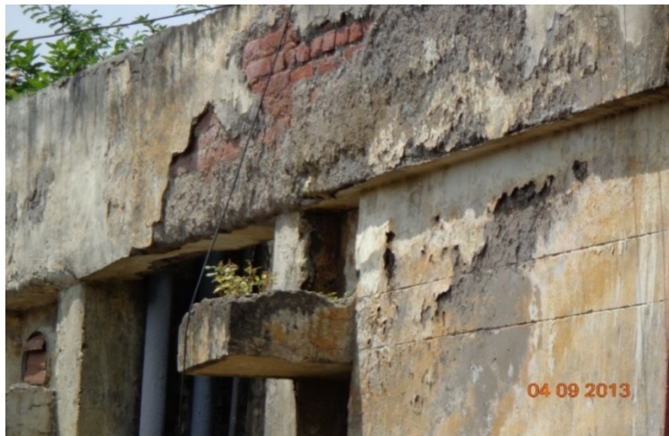
MAJOR - DAMAGES OF PLASTERING
