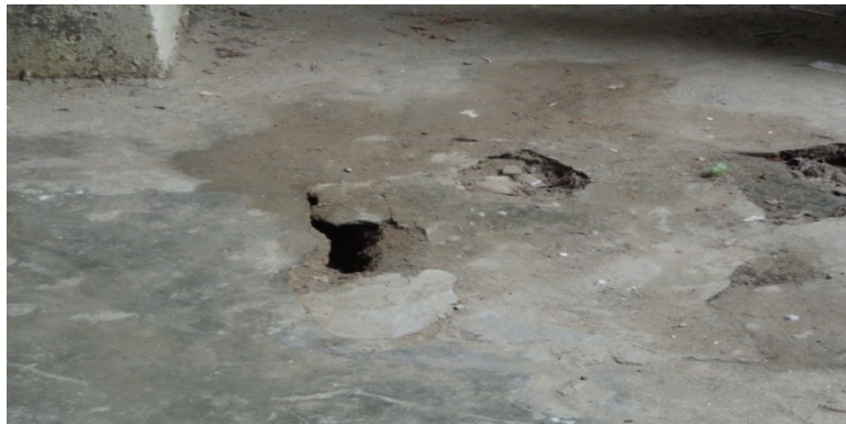
MAJOR DETERIORATION OF FLOORING
