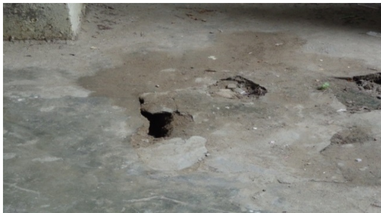
Fig.-4.17 Defect of concrete Flooring
