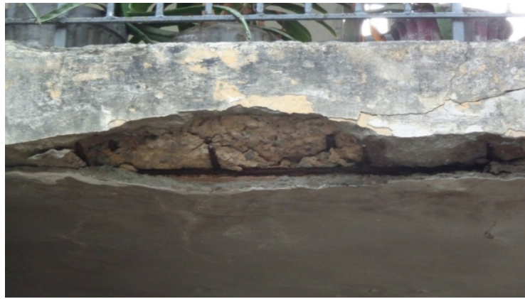
MEDIUM DETERIORATION OF RCC SLAB
