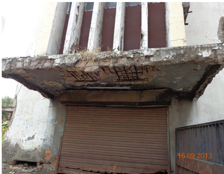
Fig. -1 Unattended repair works and poor maintenance of a building
