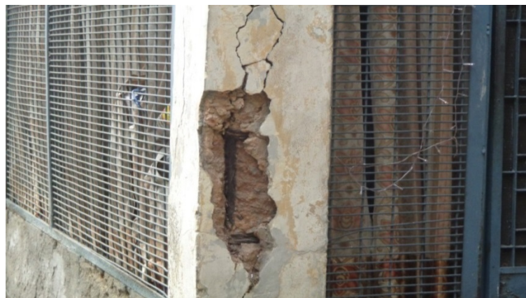
MAJOR DETERIORATION OF RCC COLUMN
