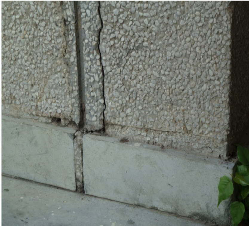
Fig. - 4.6 Vertical crack at joint
