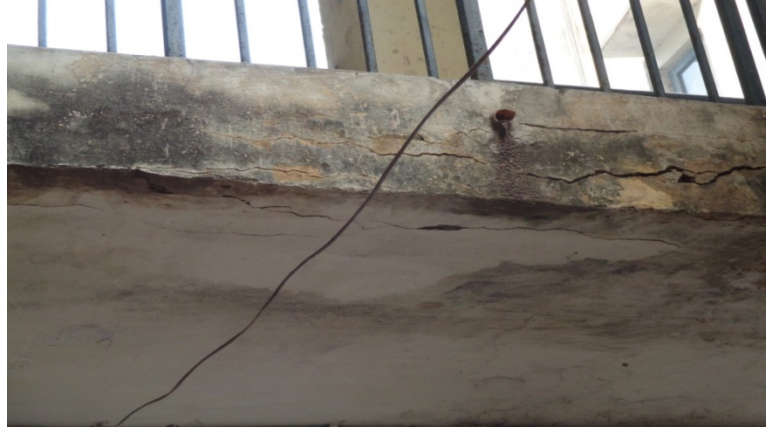
MINOR DETERIORATION OF RCC SLAB
