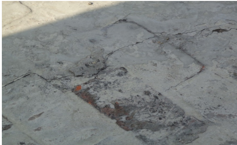
MEDIUM DETERIORATION OF BRICK FLOORING
