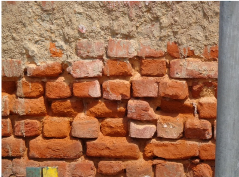
Fig. - 4.7 Loose or crumbling mortar
