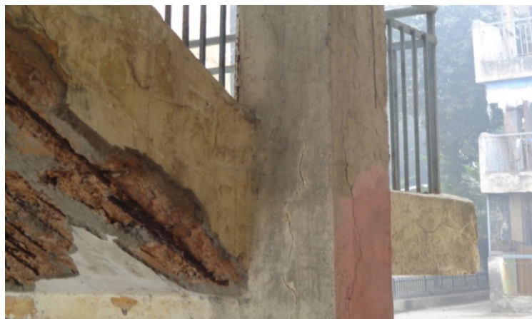
MAJOR DETERIORATION OF RCC SLAB
