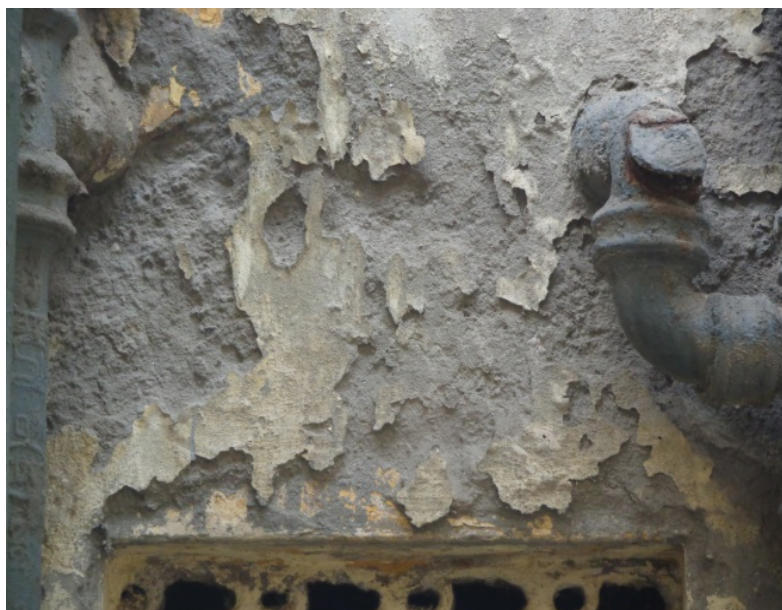
Fig.4-12 Plastering deterioration due to dampness on walls
