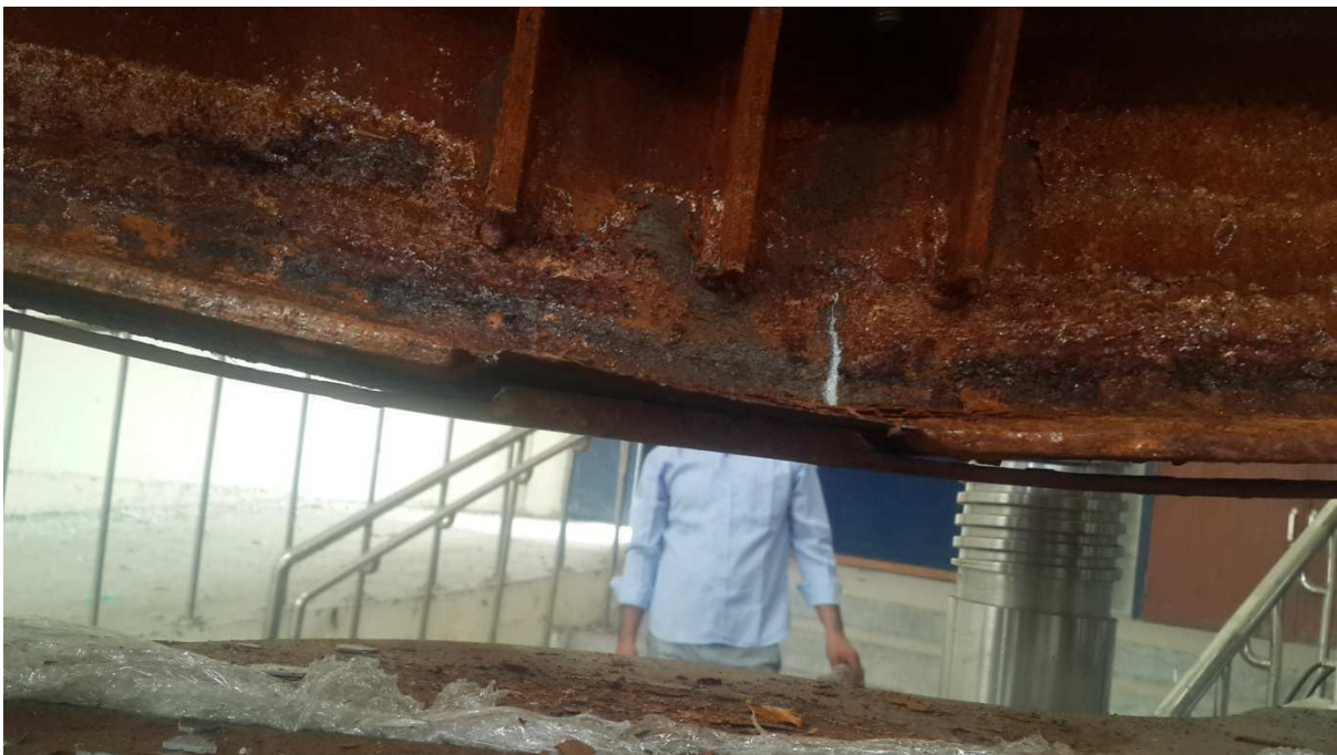
Figure 25 e): Enlarged views of Beam 6 after test showing mode of failure complete steel and adhesive interface debonding failure.
