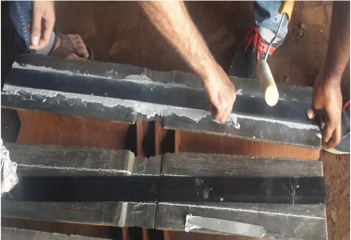
Figure 19: Image Showing Typical CFRP Strengthened Beam without End-Anchor Plates during Application of CFRP Sheets.
