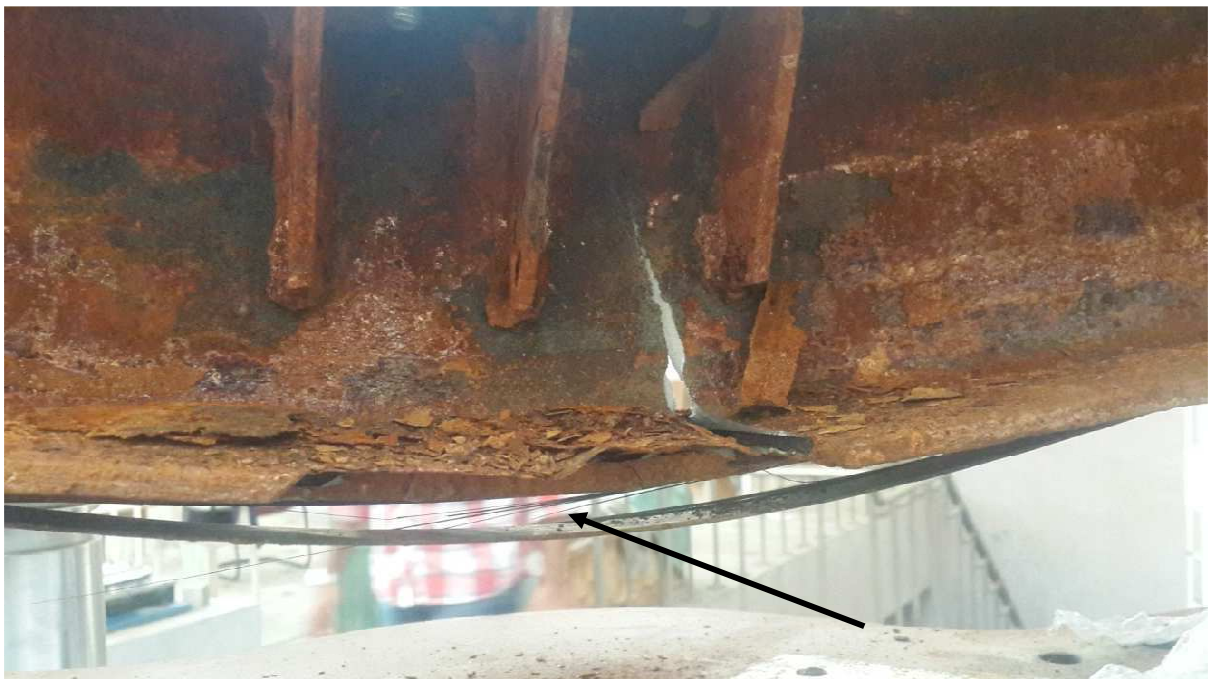
Figure 25 g): Enlarged views of Beam 8 after test showing mode of failure CFRP tensile rupture.
