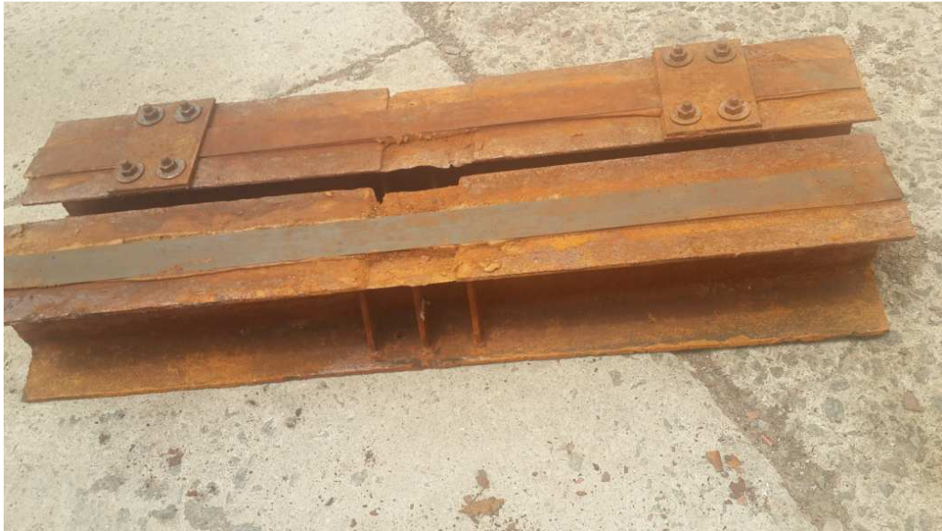
Figure 24 c) : Beam 6 and Beam 9 after exposure in saline water tank for 30 days and giving daily one wetting-drying cycle.
