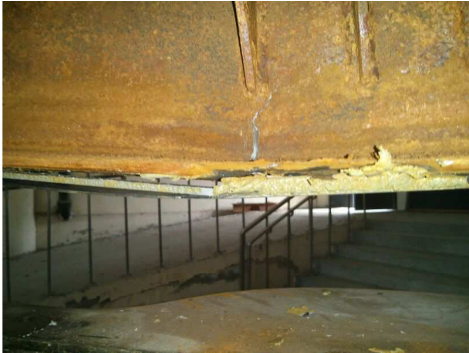
Figure 25 b): Enlarged views of Beam 3 after test showing mode of failure intermediate steel and adhesive debonding.
