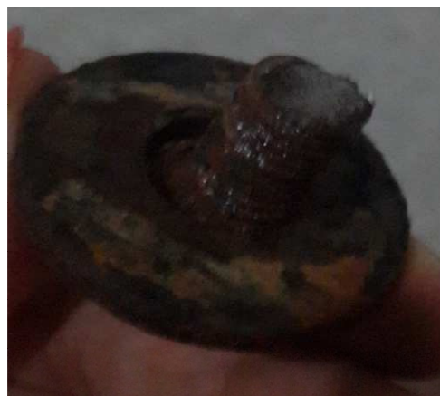
Figure 26: Image showing the failed bolt of end anchor arrangement of beam 9
