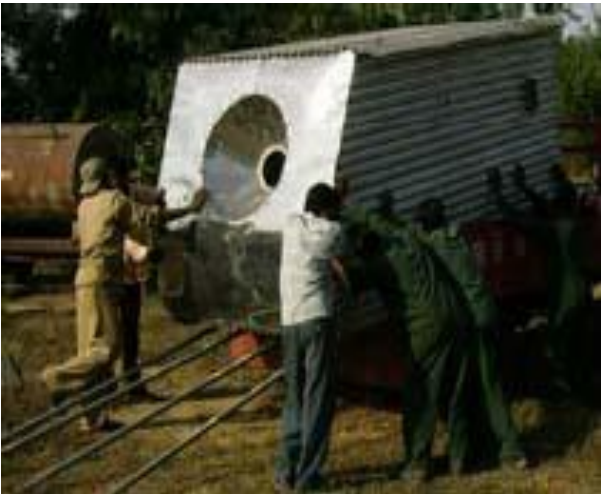
Fig. 4.11 : Chamber (front) arrives in; Focal-opening 240 mm diameter, Connection for air-blower at the side
