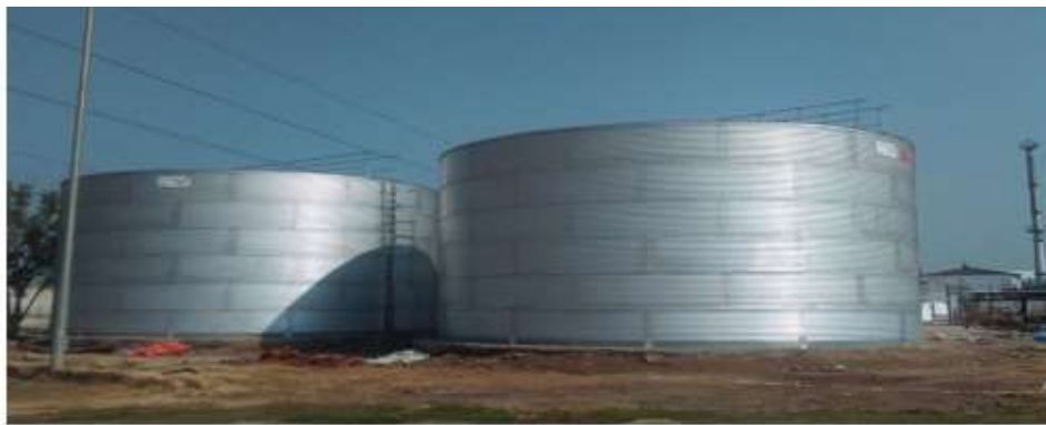
Fig. 10: Effluent Storage Tank
