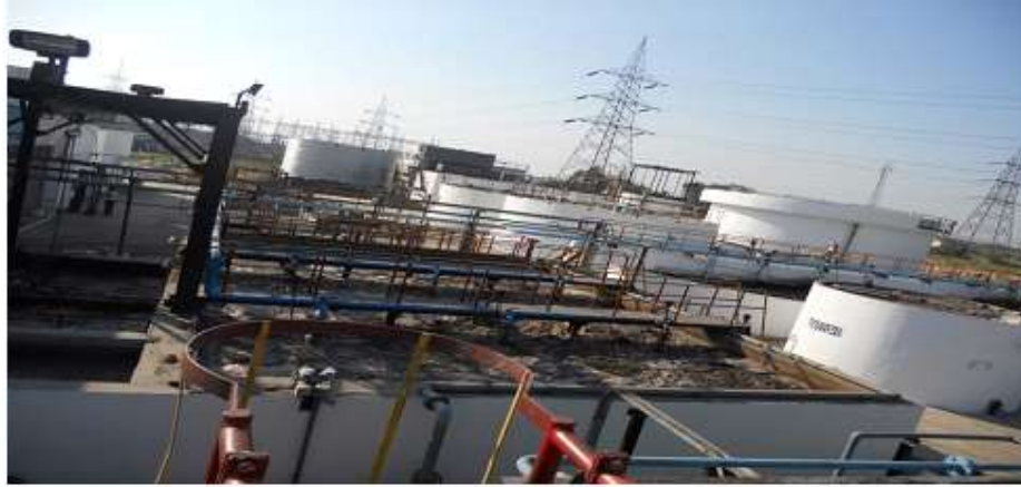
Fig. 6: Arial View of ETP Plant. Capacity-900 KLD
