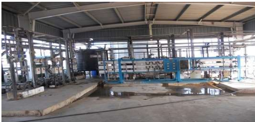
Fig. 8: RO unit of ETP Plant. No. of RO Streams 1. RO Permeate Flowrate / Stream-13.13 m 3 /hr
