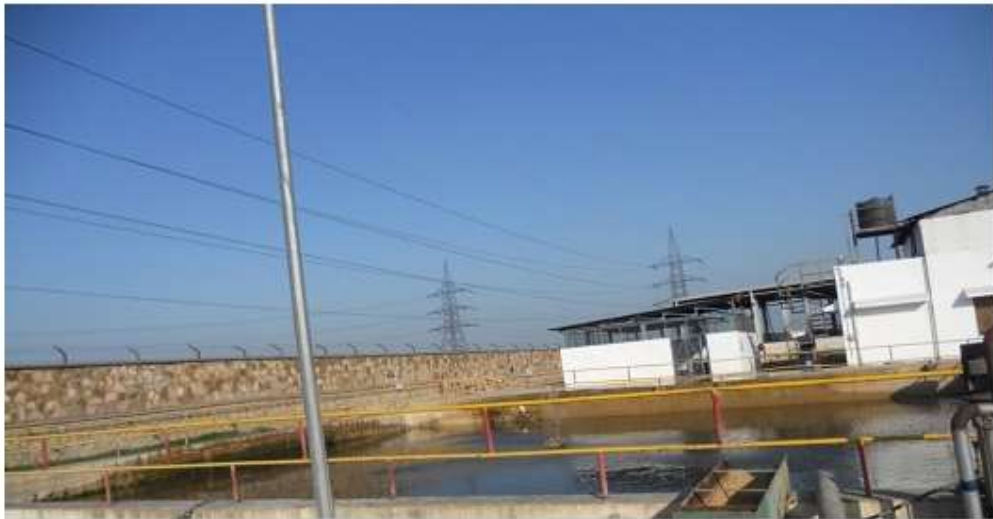
Fig. 9: Treated Water Tank. Capacity of Tank-550 m 3
