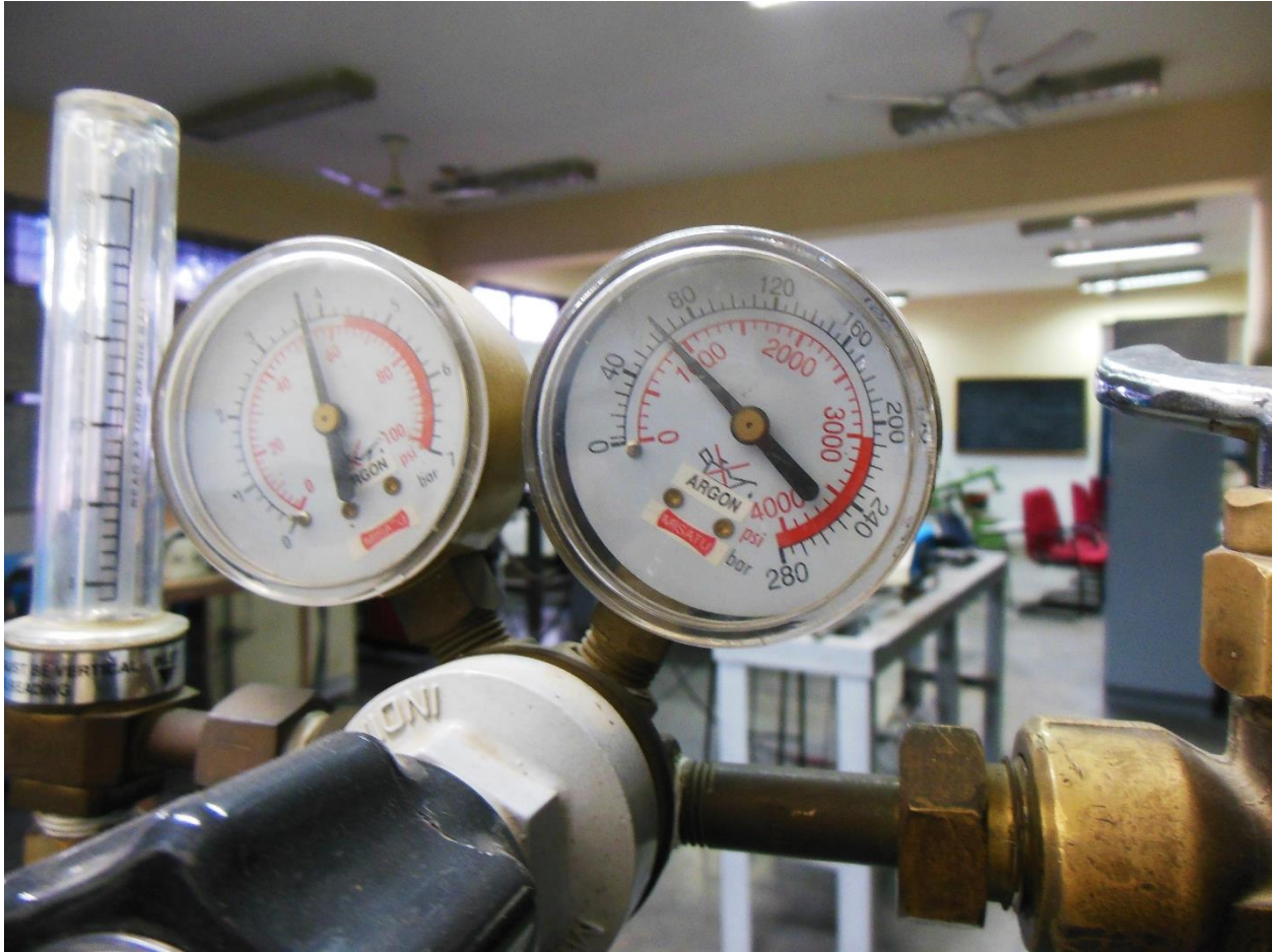
Figure 3. 6: Gas flow rate meter
