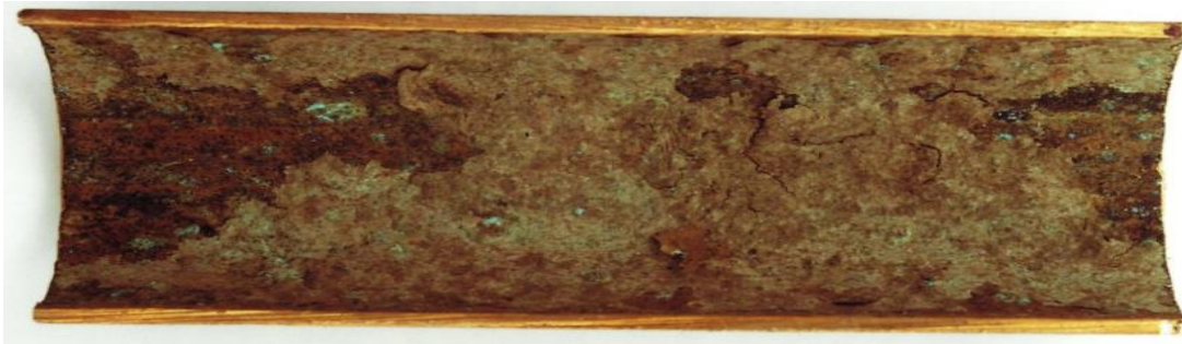
Figure 1.5: Condenser tube with residue of biofouling.[14]
