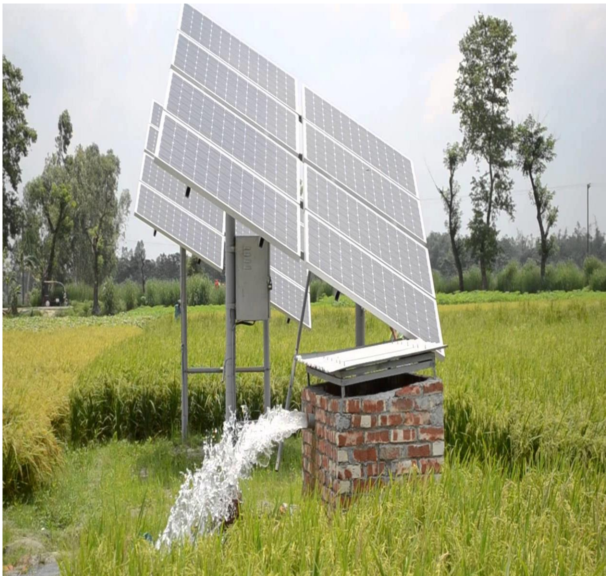
Fig 10: Solar Water Well
