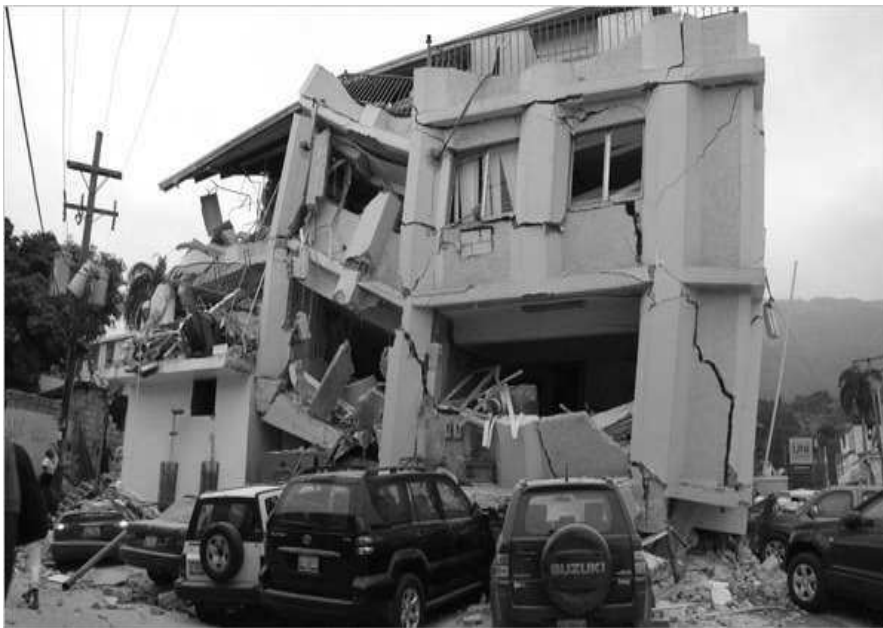
Fig.1.2: Failure of an URM building during 2010 Haiti earthquake
