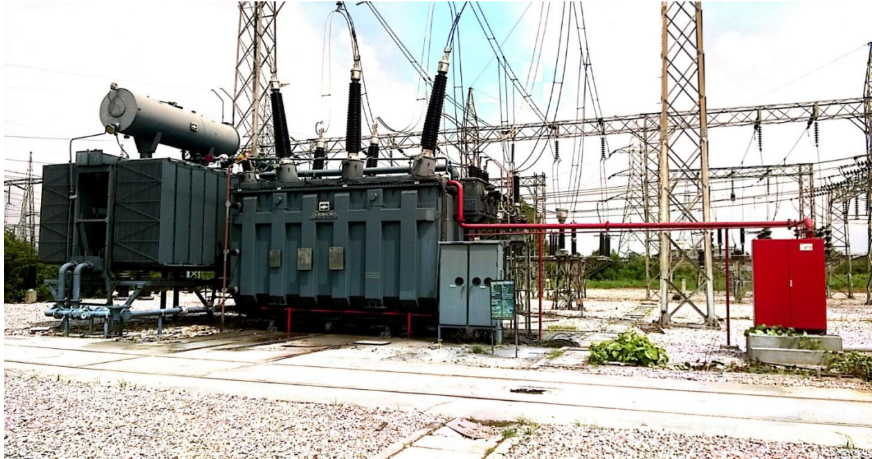
Figure 1.4: Transformer Installed at 220 kV Substation
