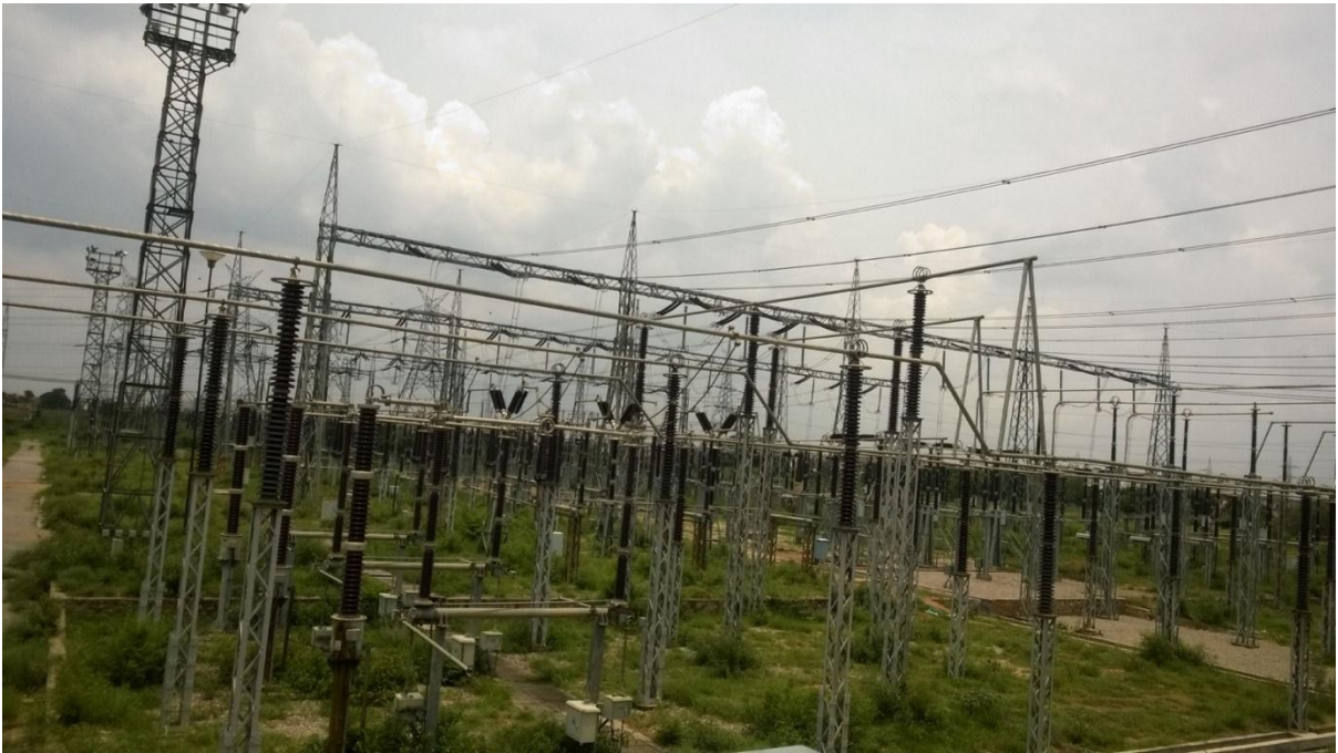
Figure 1.3: 220kV switch yard
