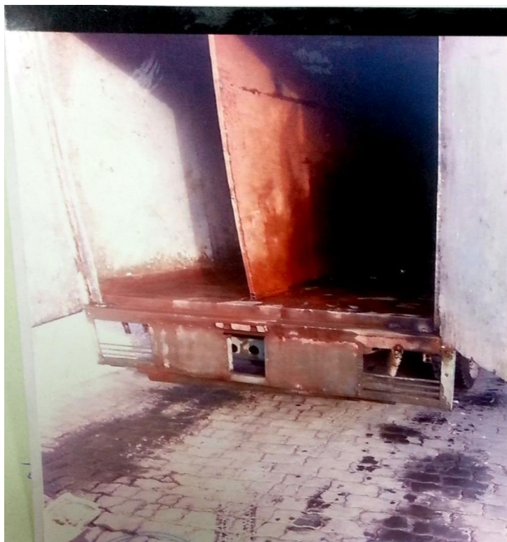
Figure 5.8 Partition in waste carrying vehicles
