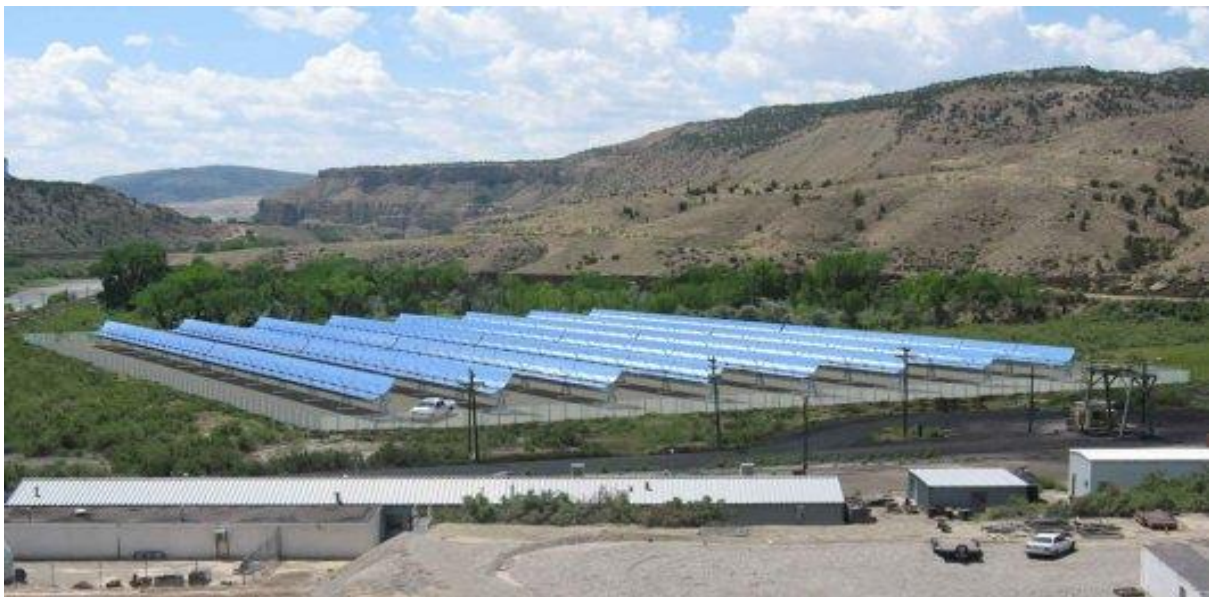
Figure 2.6 Solar-coal hybrid combined-cycle Cameo plant[25]
