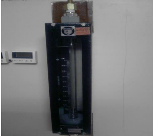
Fig.4.7 Flow meter/Rota meter
