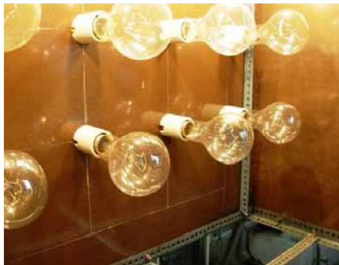
Plate 3.7: Load Bank (rear side)
