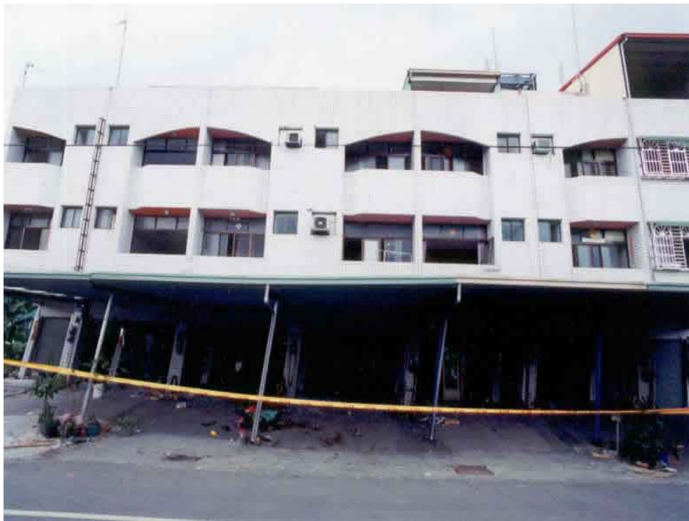
Fig. 1.3: General mode of failure in OGS buildings
